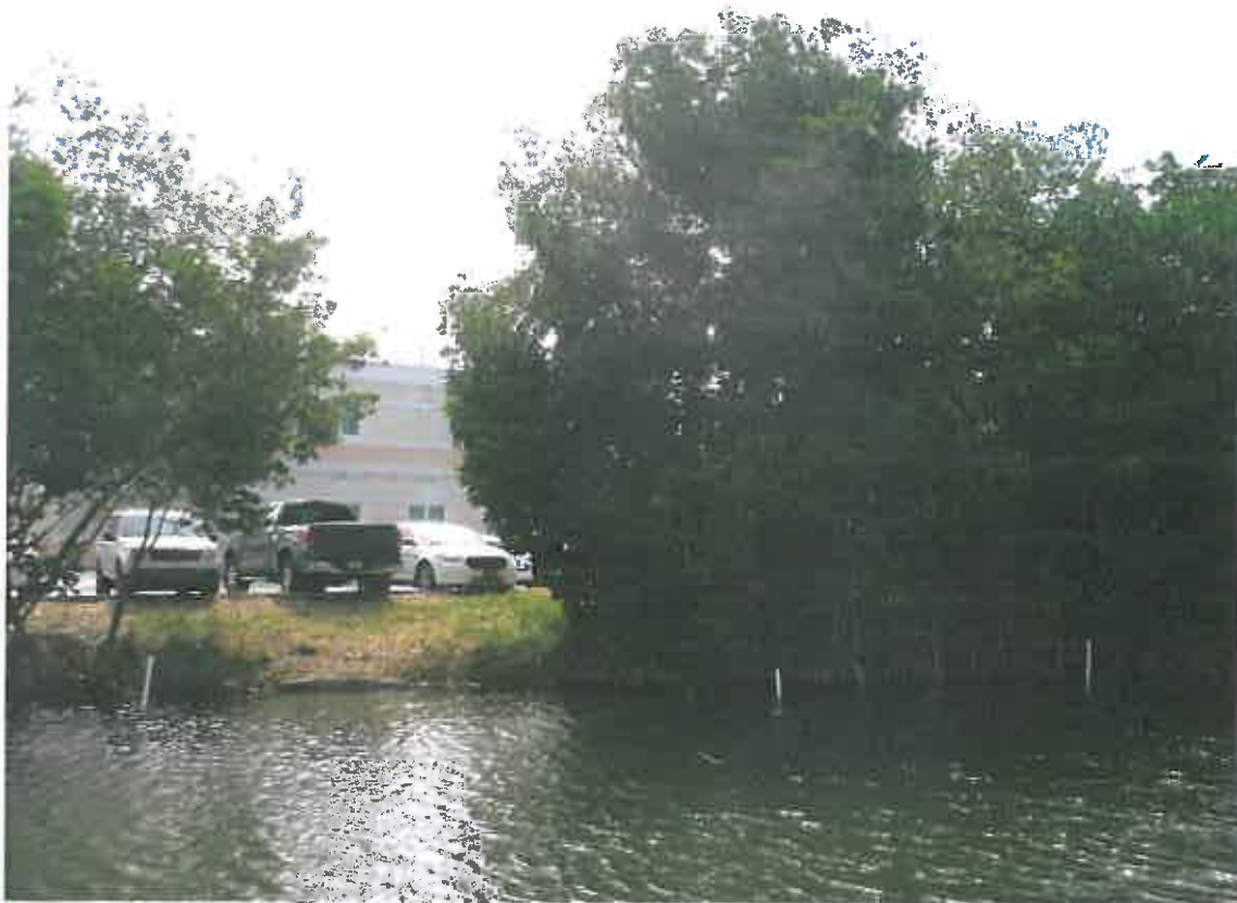
Standing on the sidewalk along Jose Marti Blvd looking east toward Key West Police Department property at existing culvert area.
