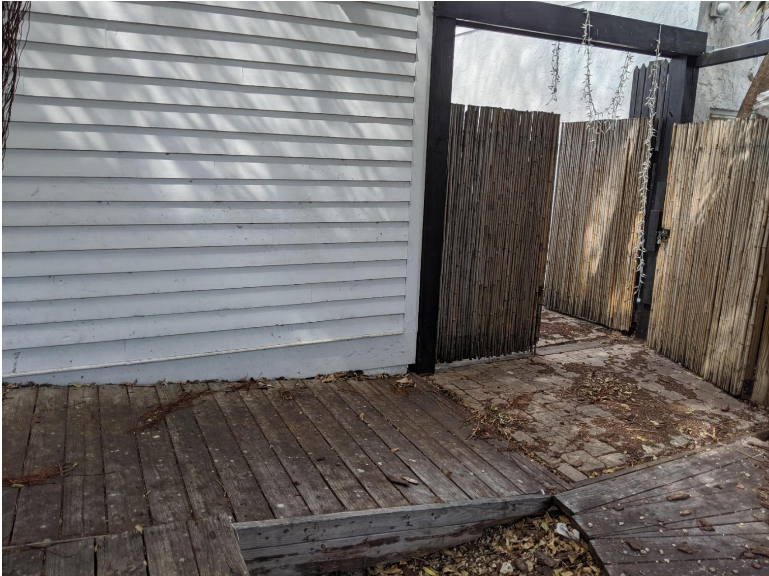
Entering the front yard, going through the side yard to the rear yard is a ADA accessible ramp to the interior first floor of the structure.
