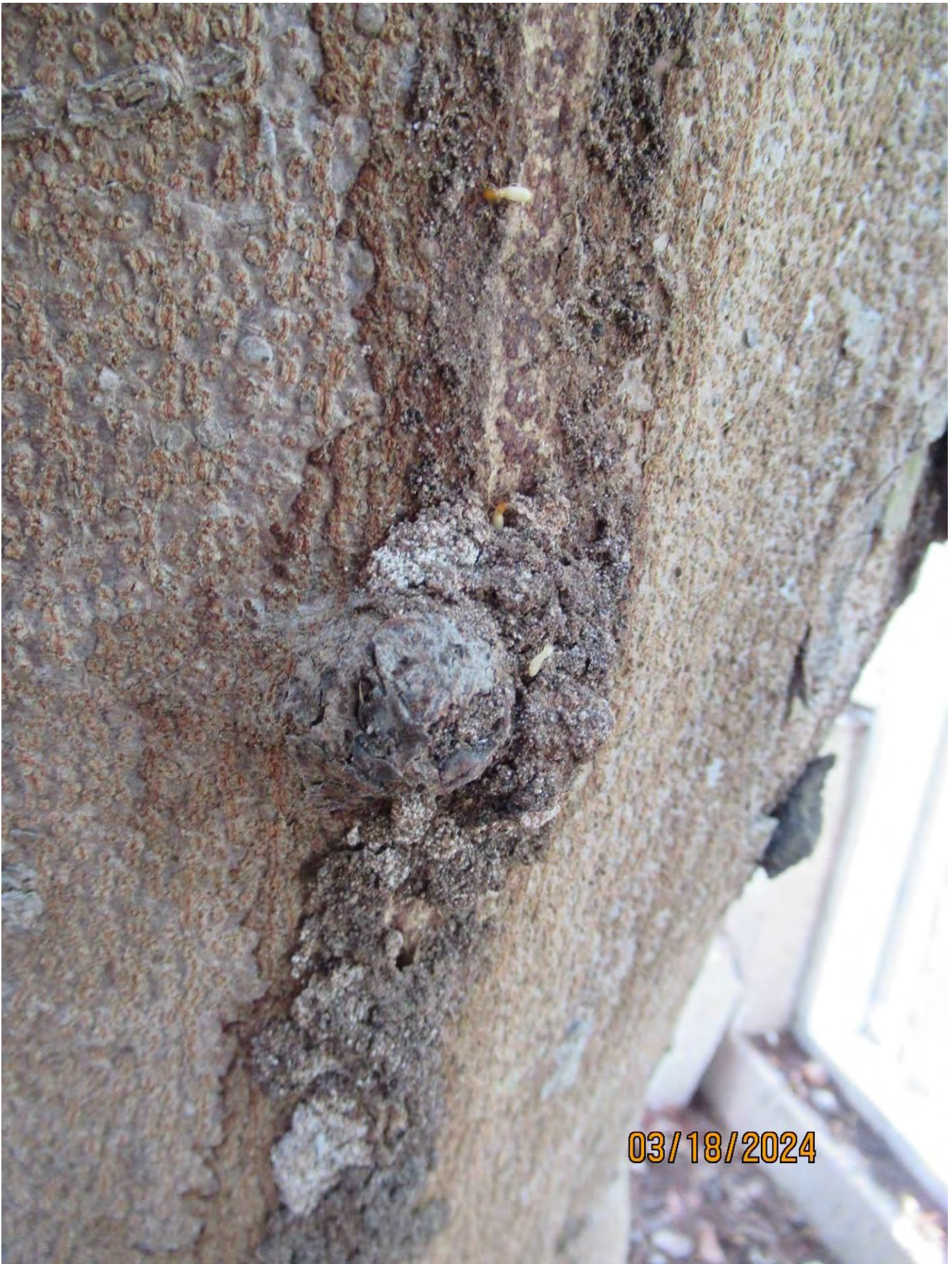
Photo showing active termites in mud trail.
