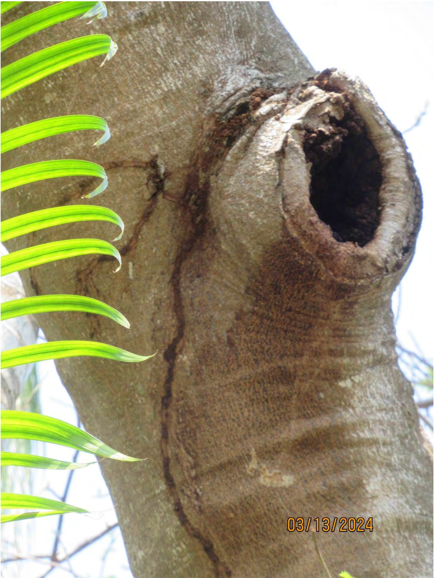
Close up photo of decay area and subterranean termite trail, view 2.
