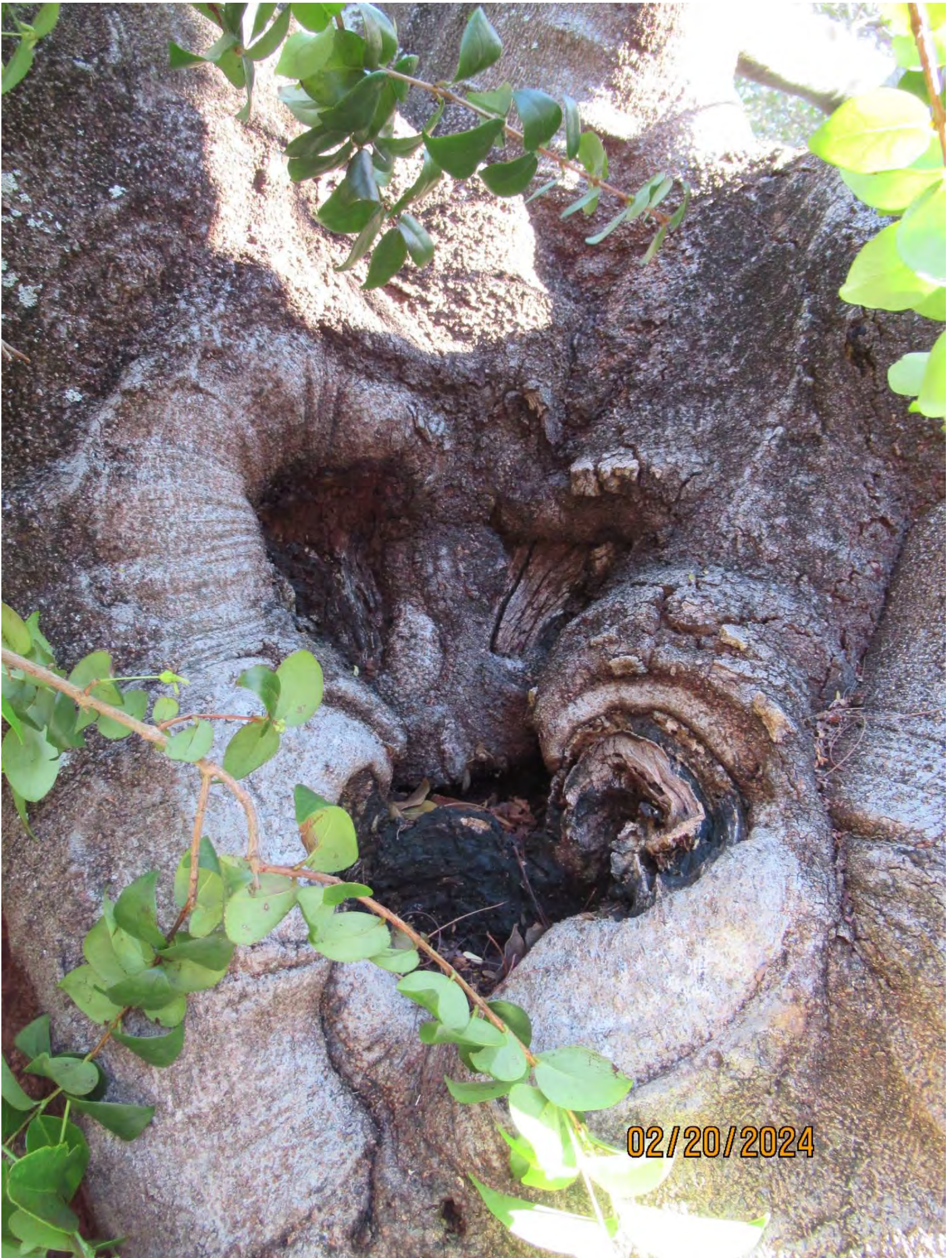
Photo of fungal growth, decay area.
