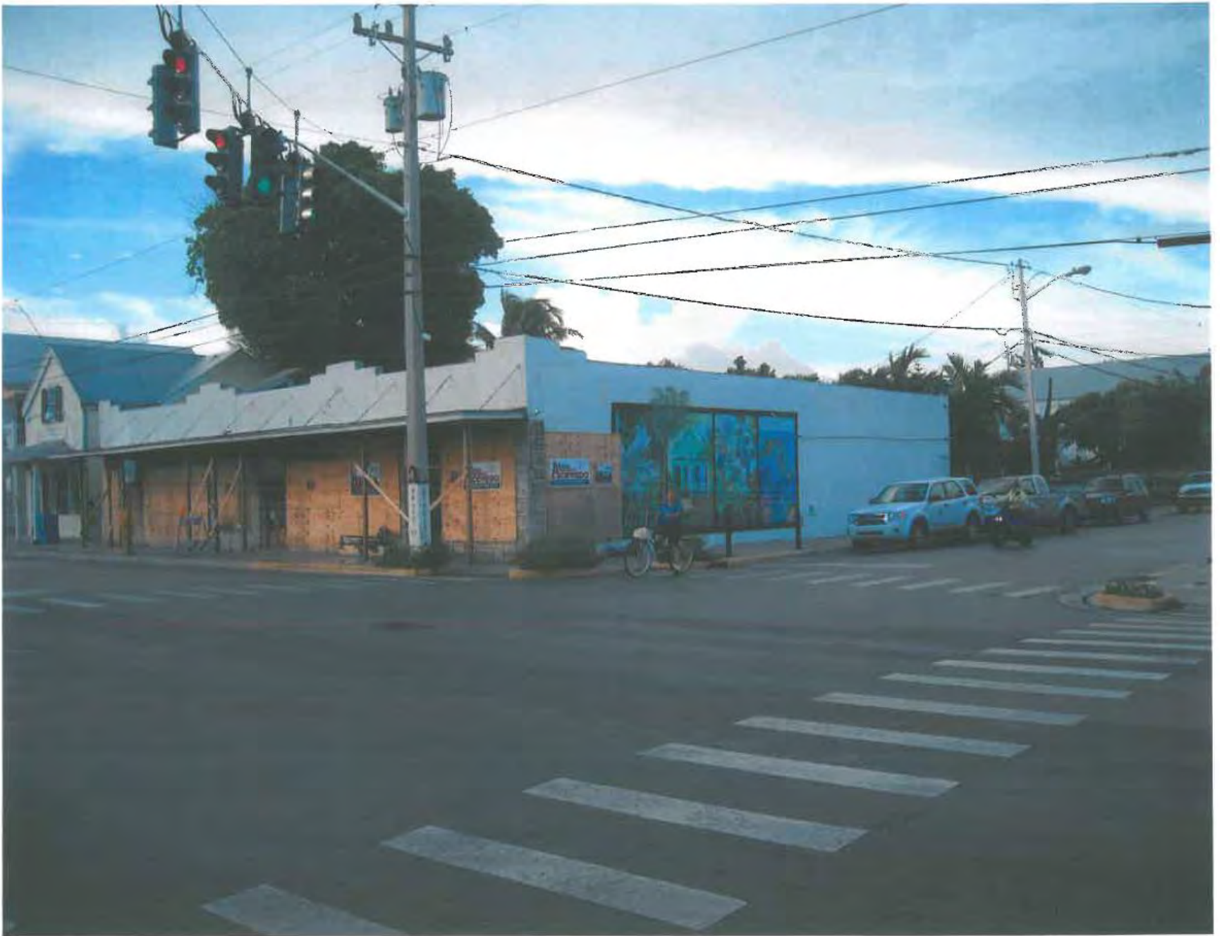
Building after 2008 fire.
