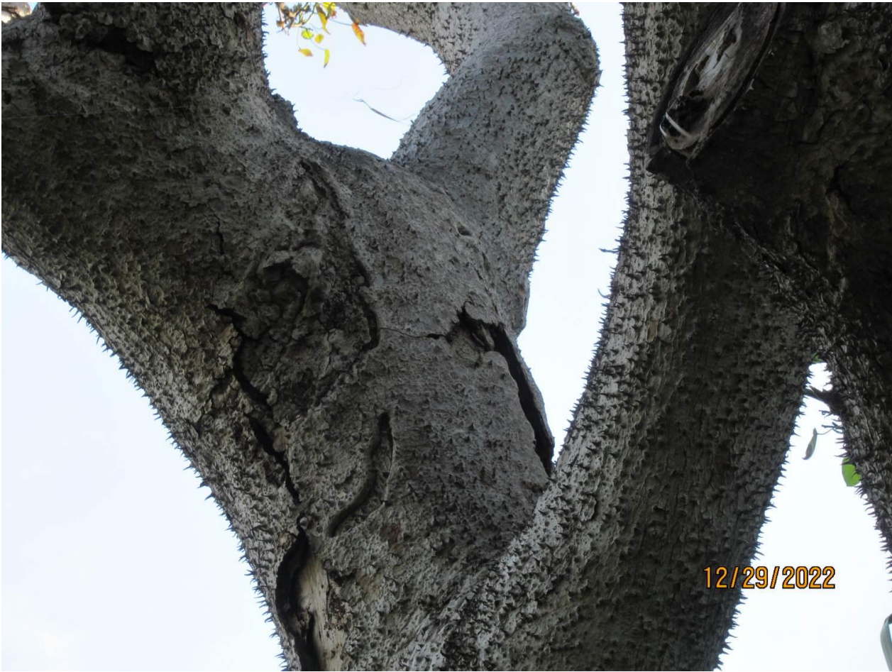
Photo showing decay area in canopy branches, view 1.
