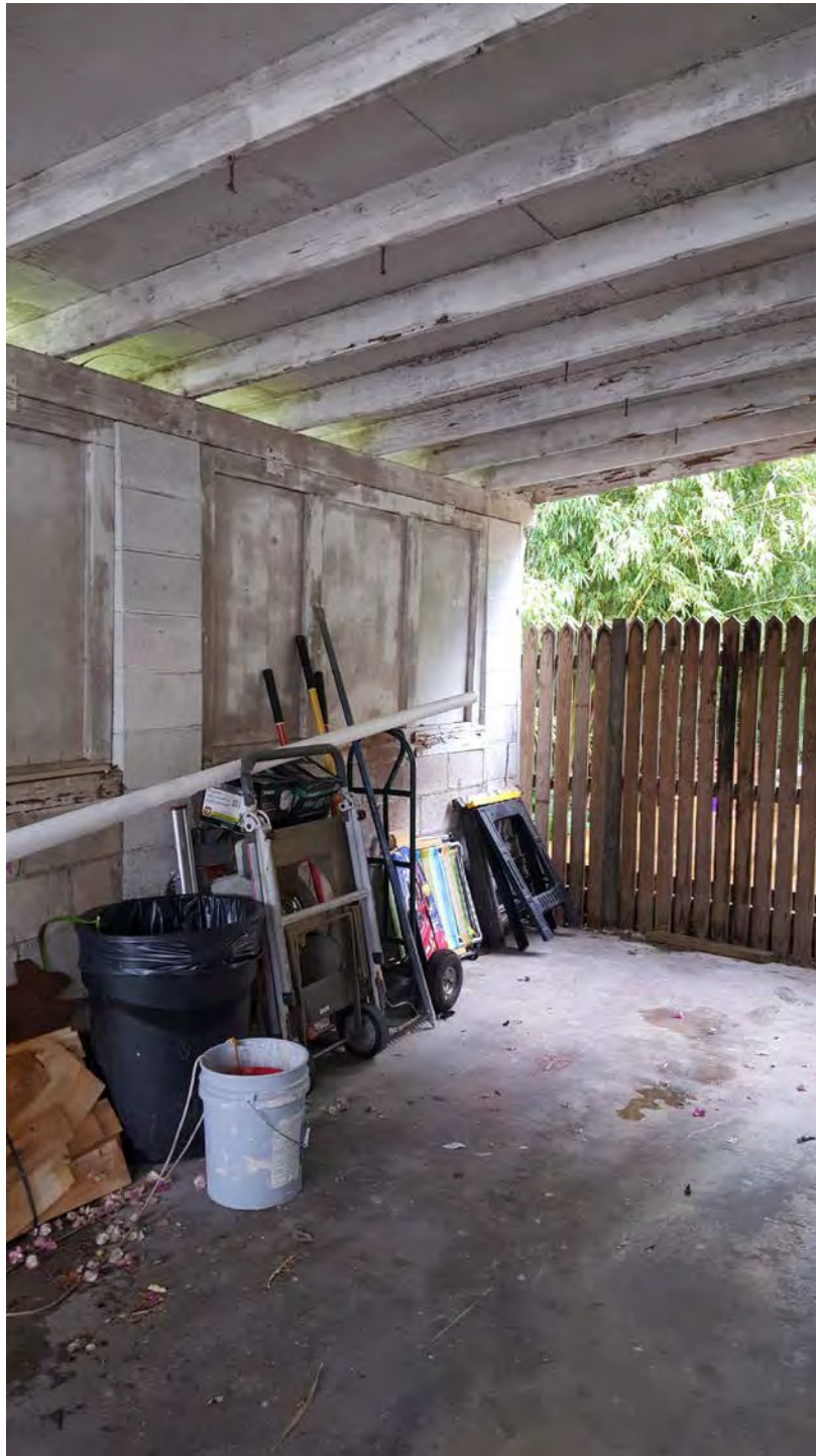
1212 Margaret Street – View of carport illustrating simple construction and concrete block supporting wall
