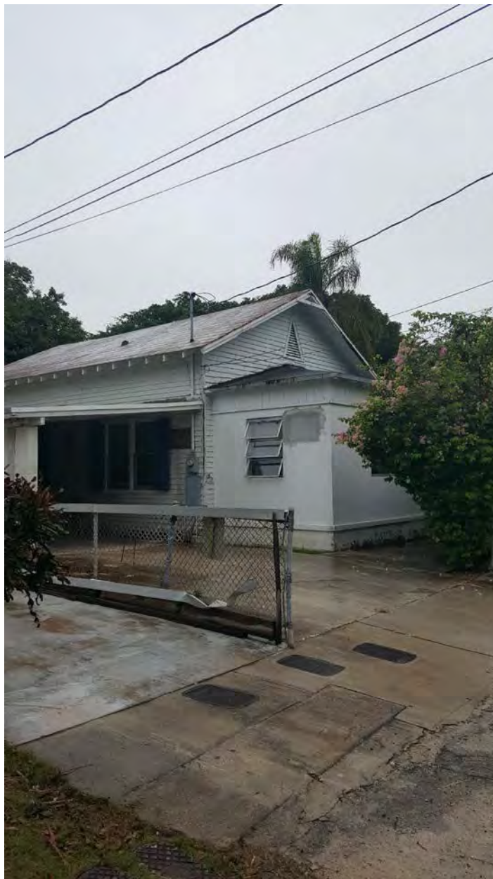
1212 Margaret Street – View from Front Left Illustrating Former Front Porch with Stucco Façade
