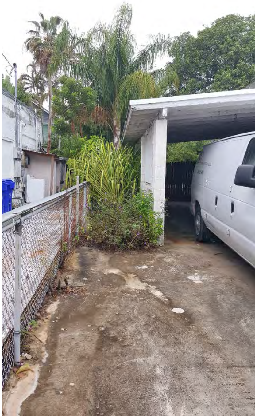
1212 Margaret Street – View of carport illustrating simple construction and concrete block supporting wall
