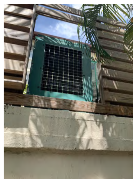
EXISTING GENERATOR VENT
