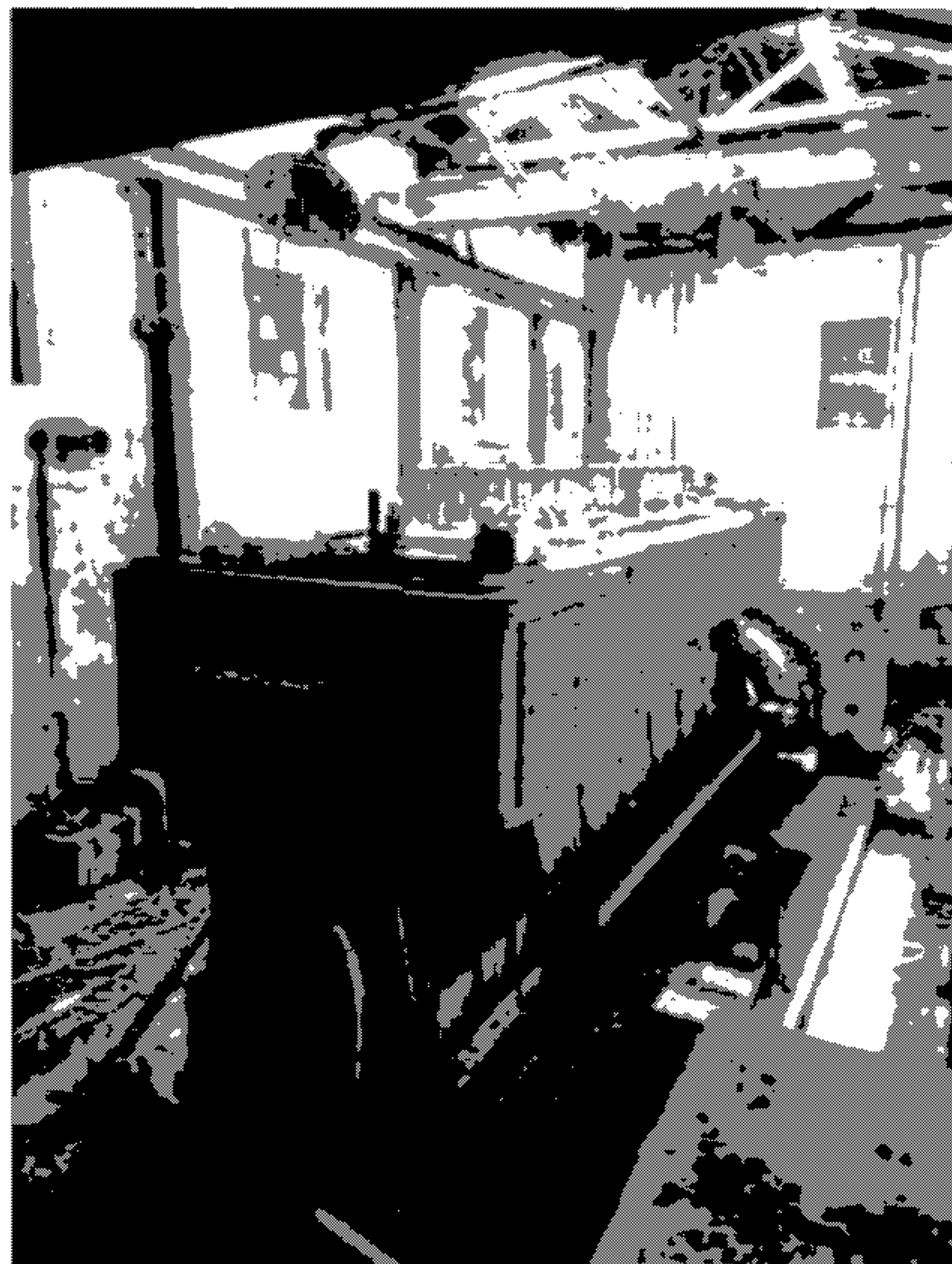
Nordberg Dynamo generator in Building 4
