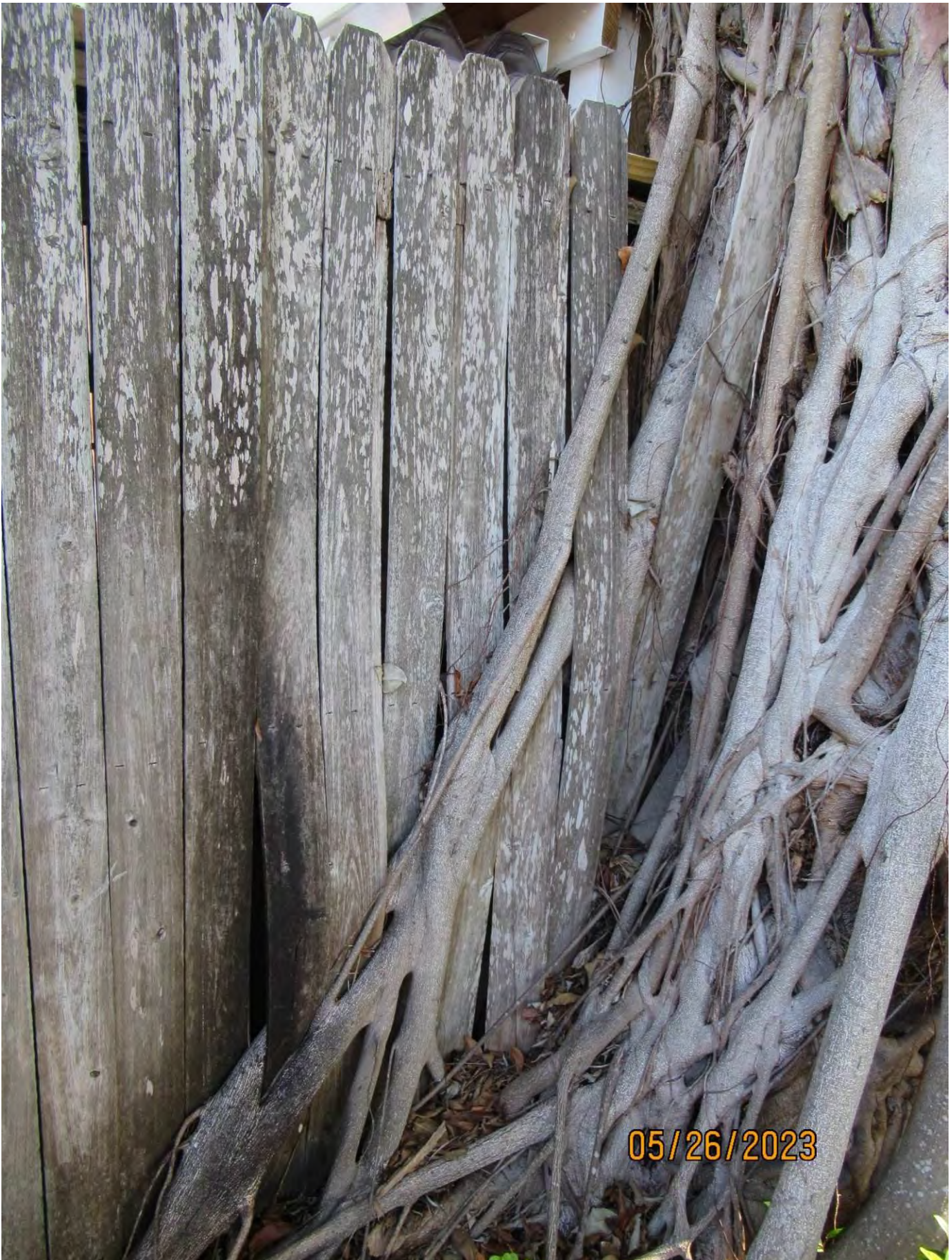
Close up photo of tree trunk and aerial roots impacting property line fence, view 2.
