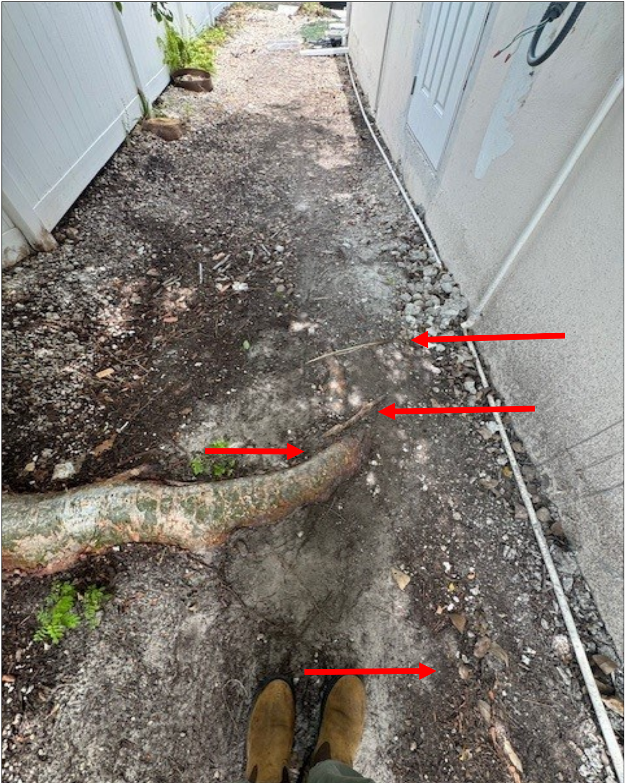
If left in place, roots will eventually reach the structure and may do damage. House appears to be on a slab.
