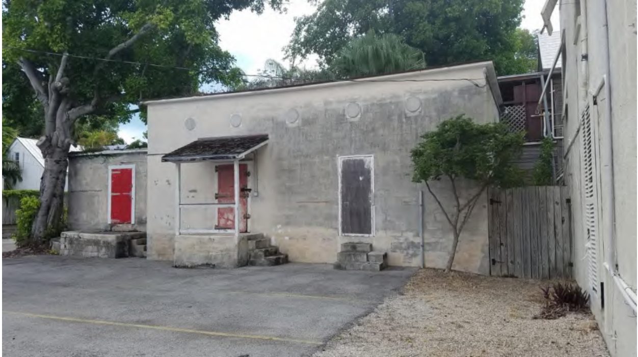
Building 4, a concrete 'ice house' building at rear or parking area. Date from circa 1948-65. No work except reroofing.
