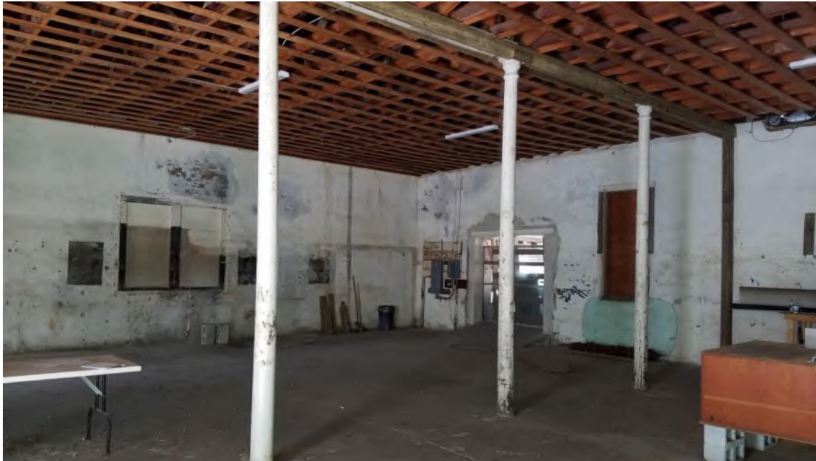
General view of the interior of the 1891 building 1. The cast iron columns are original and shall be restored.
