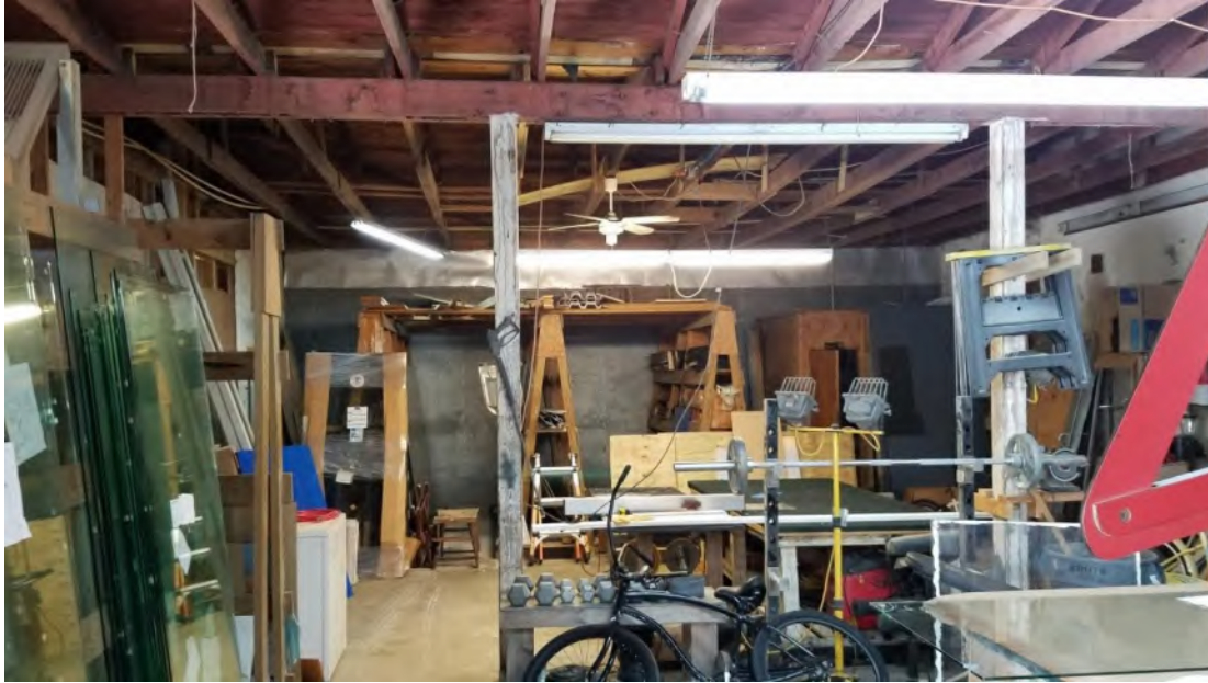
General view of Building 3 interior, a rear addition to Building 1. This addition was constructed circa 1948-65. Finishes include concrete floors, plywood/hardboard walls, and open roof trusses.
