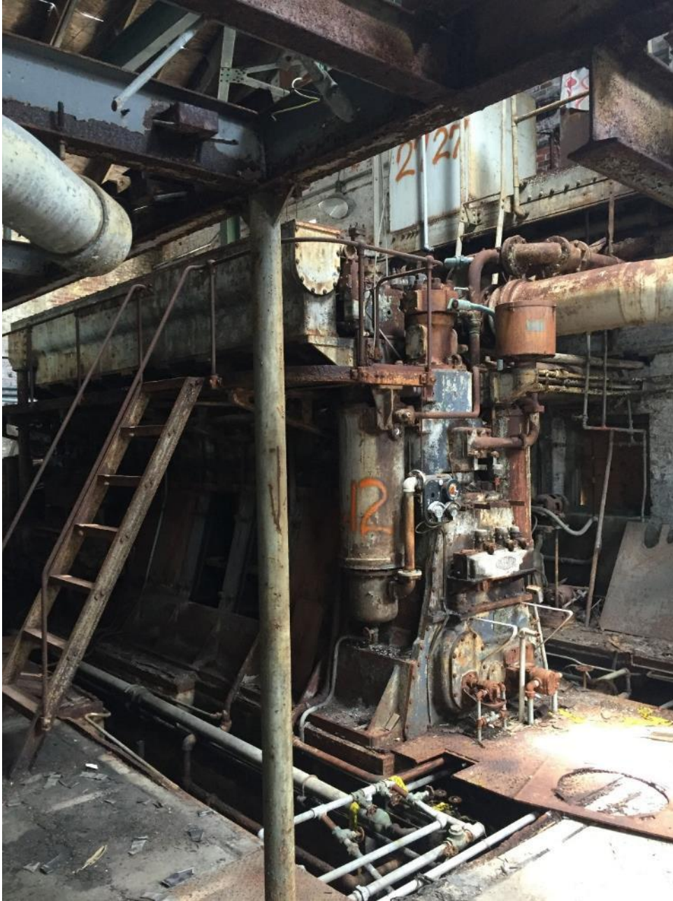
PHOTO 2: Inactive generator inside buildings at the Site
