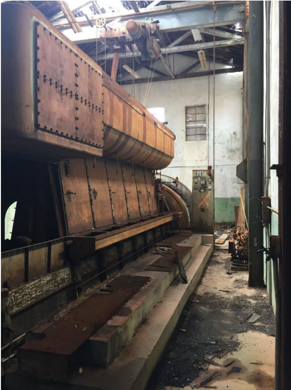
PHOTO 11: Interior of buildings at the Site showing an inactive generator
