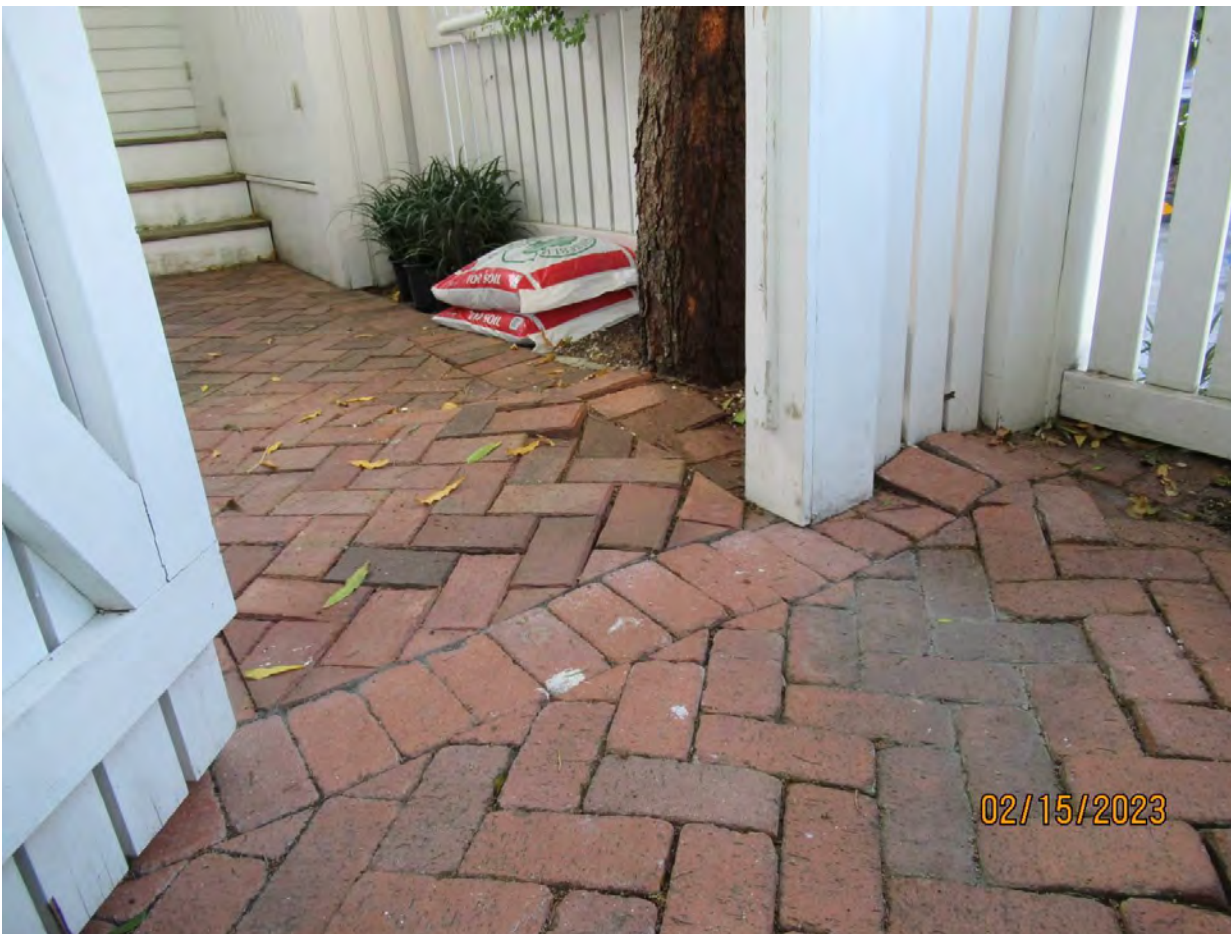
Photo showing base of tree, view 1.
