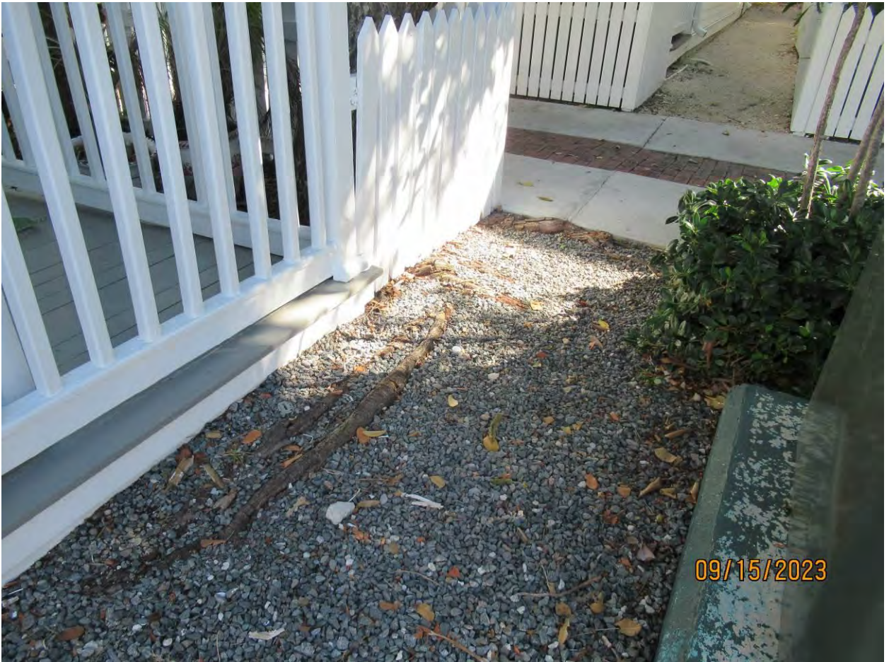
Photo showing base of tree area/ roots and impacts to fence.
