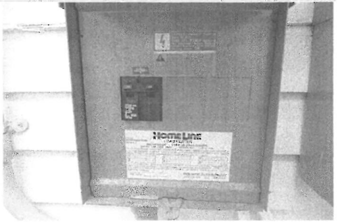
Disconnect -60 amp typical all units except #3
