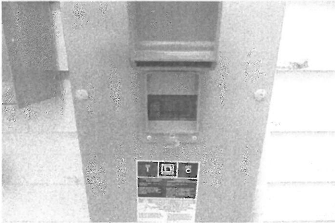
Disconnect 100 amp - Unit #3
