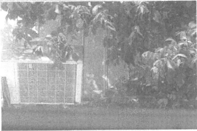
Ductless Mitsubishi system
