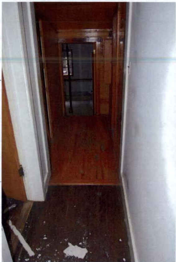
View looking from interior of historic house to the non historic additions. First addition is 5" below historic floor, the second addition is at grade (approximately 2'-0" below historic home).
