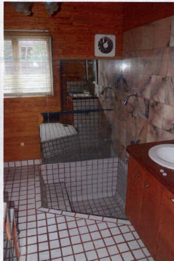
Sunken tub in non historic addition. Finished floor in this addition is 5" below historic structure.
