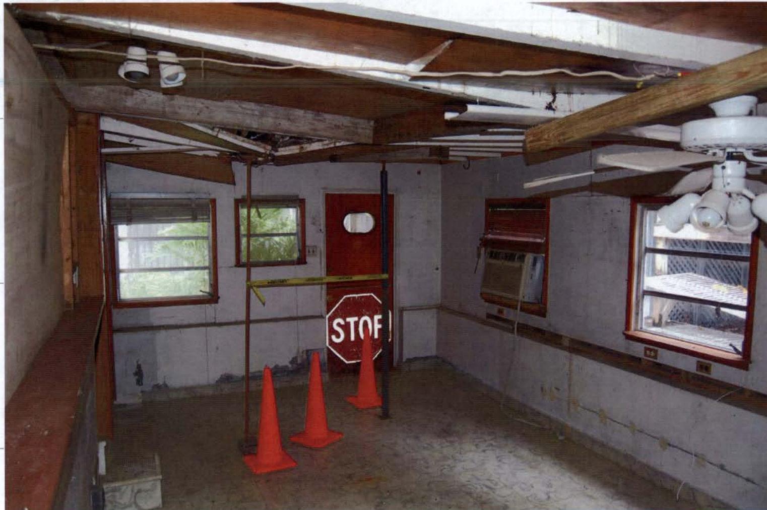
Photograph of Southernmost addition. Finished floor of this addition is approximately 2'-0" below that of the historic structure.
