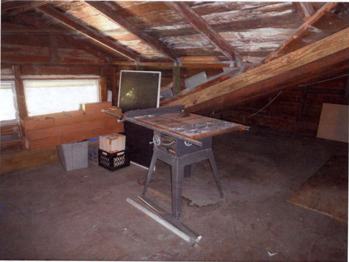
(photograph showing the use of non "historic" lumber to create dormer and hurrican clips which are non-existent at the rest of the historic roof structure)
