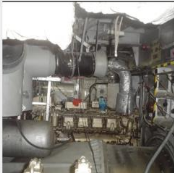
Diesel & pump machinery room
