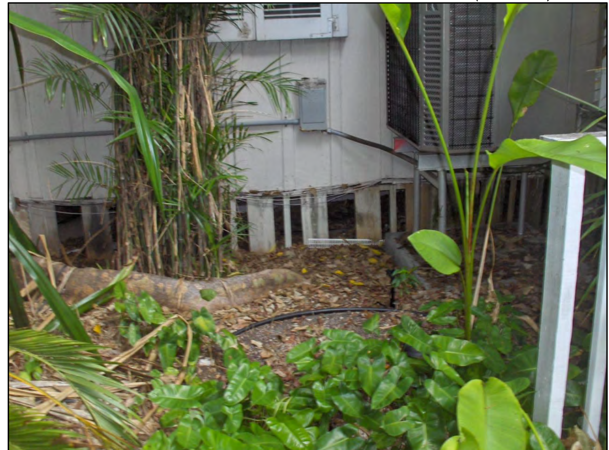
DETAIL PHOTOGRAPH SHOWING THE BOARD AND BATTEN AT HISTORIC STRUCTURE (SOUTH SIDE)
