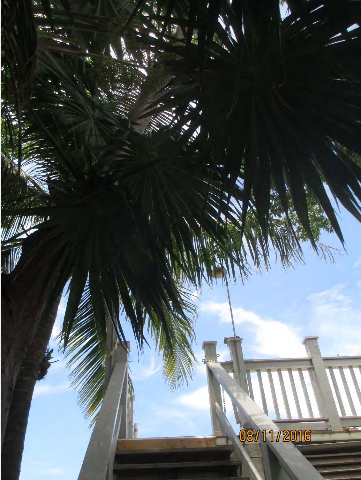
View looking up the rear stairs. Palm fronds and tree branches may need to be trimmed prior to commencement of construction work.
