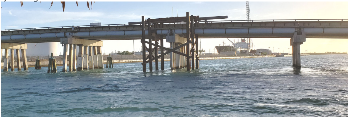
Figure 1. Front view of temporary stabilization of damaged pier. (looking westward)
