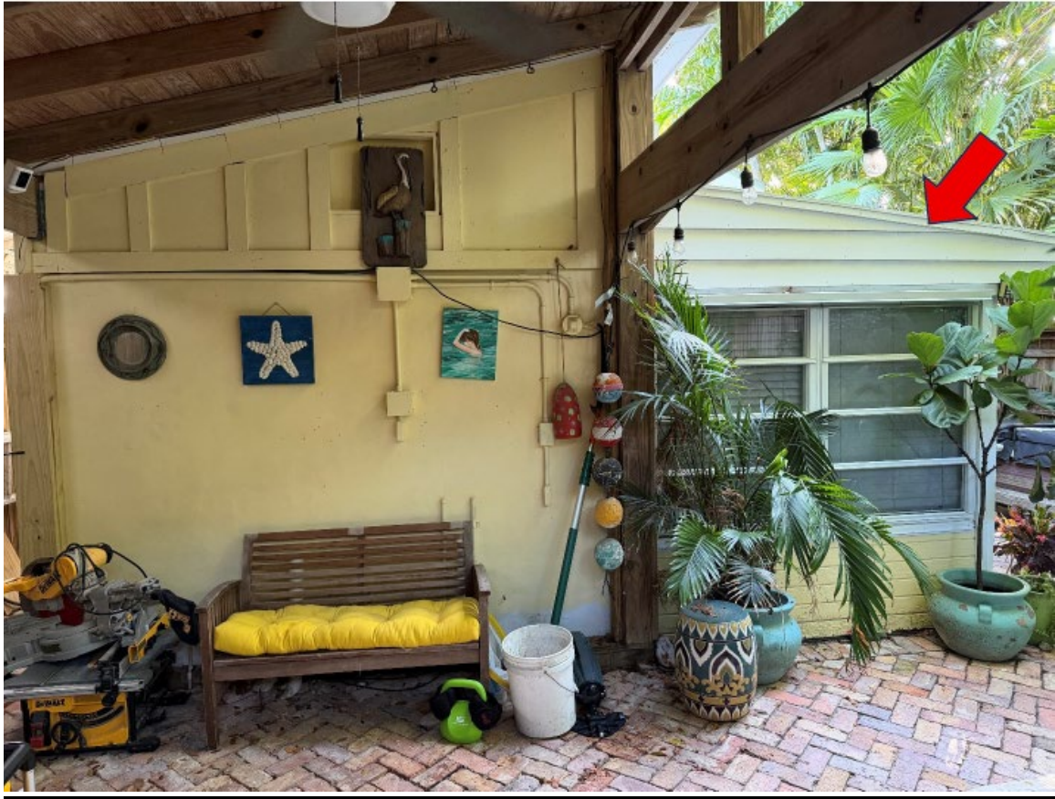
Photo of Rear of Property Under Review Showing Addition Proposed to be Demolished.
