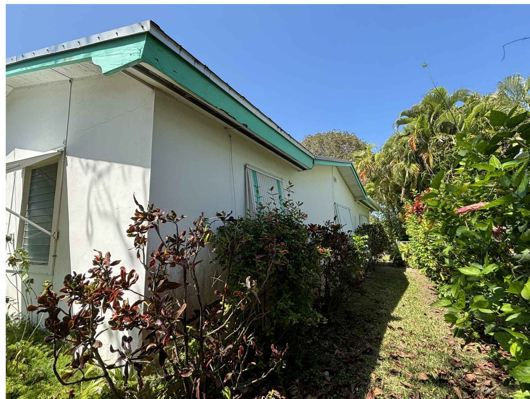
2 A8 VIEW FROM SIDE OF THE HOUSE (EXISTING EAST ELEVATION) SCALE: N.T.S.
