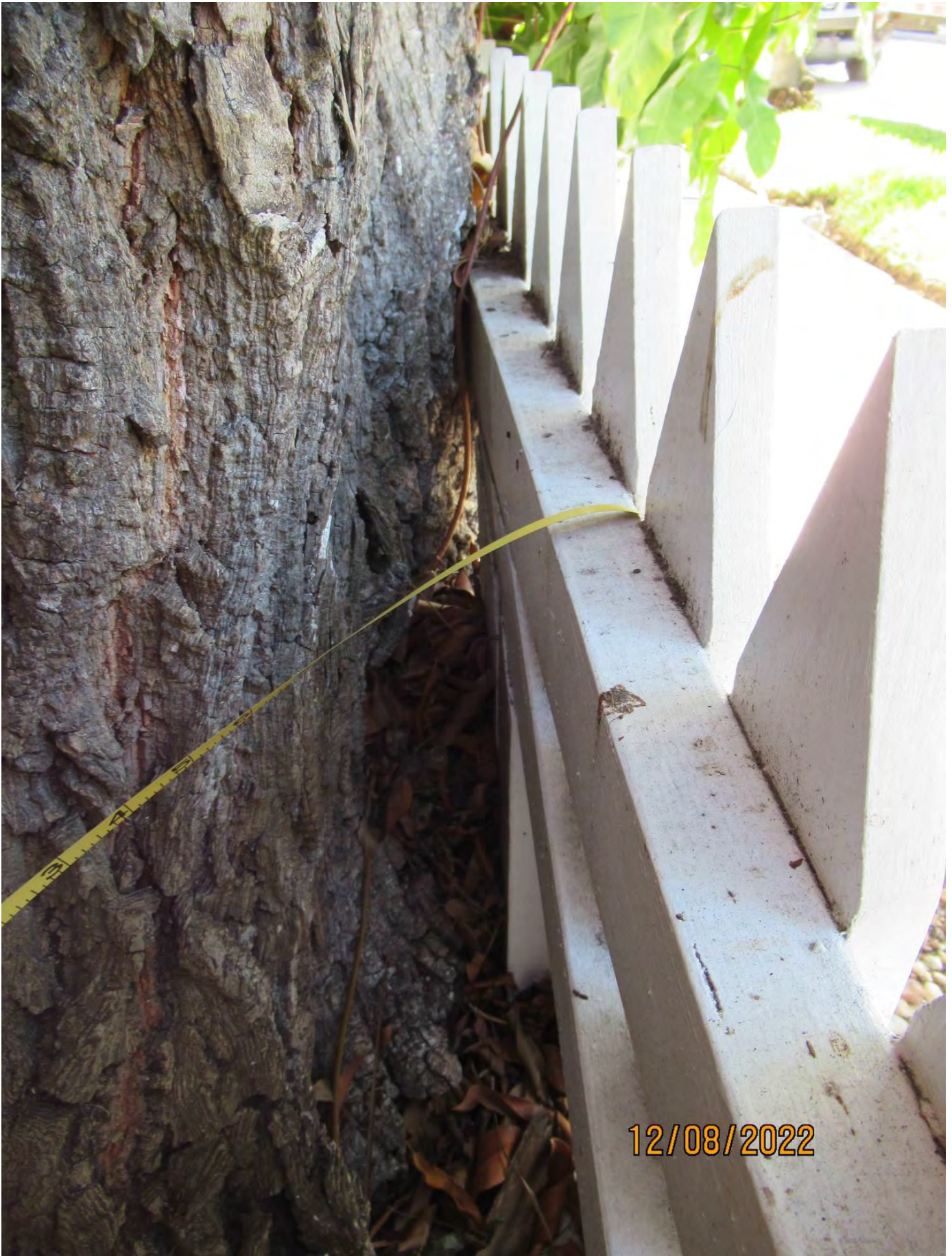
Photo showing trunk of tree in relation to sidewalk fence.
