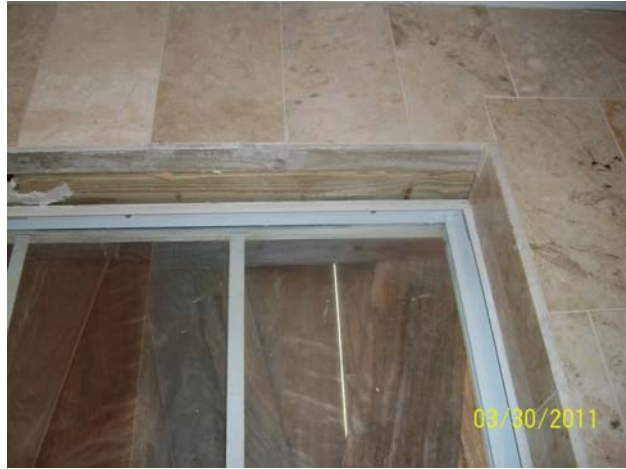
New framing for window. Window not approved by HARC
