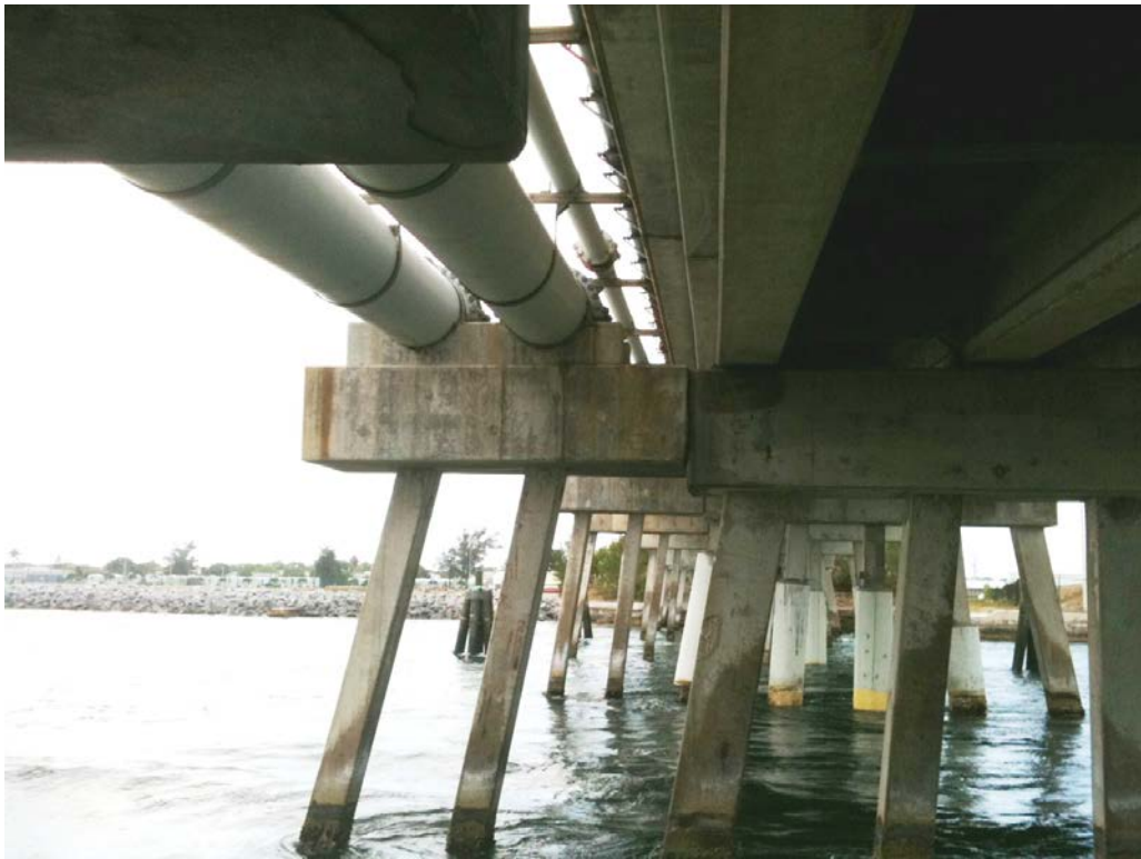
The City of Key West Sewer Bridge is the two pilings and concrete support for the two pipes on the left of the picture. It sits immediately adjacent to the Navy's roadway bridge to Fleming Key
