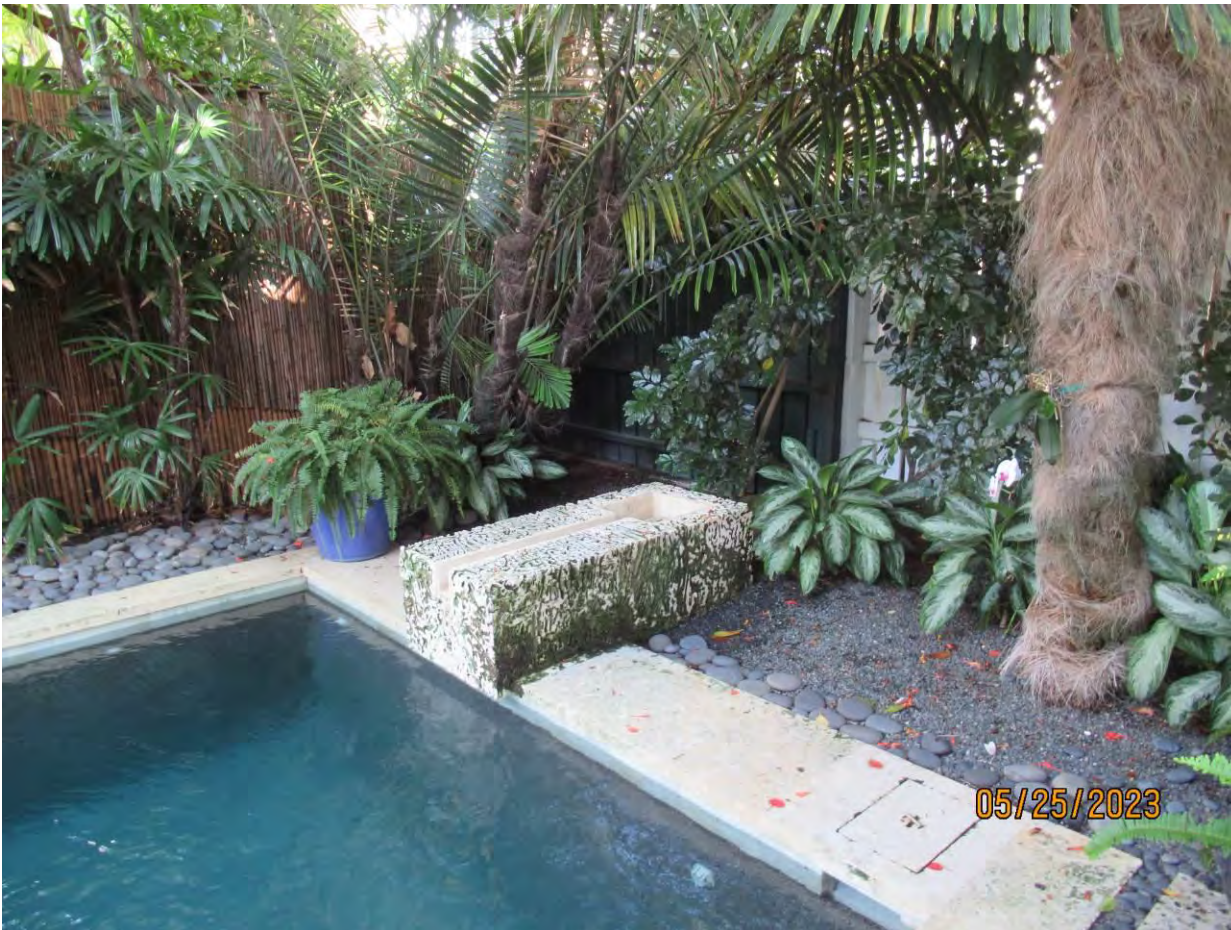
Photo of neighbor's property showing impacted area from tree roots.
