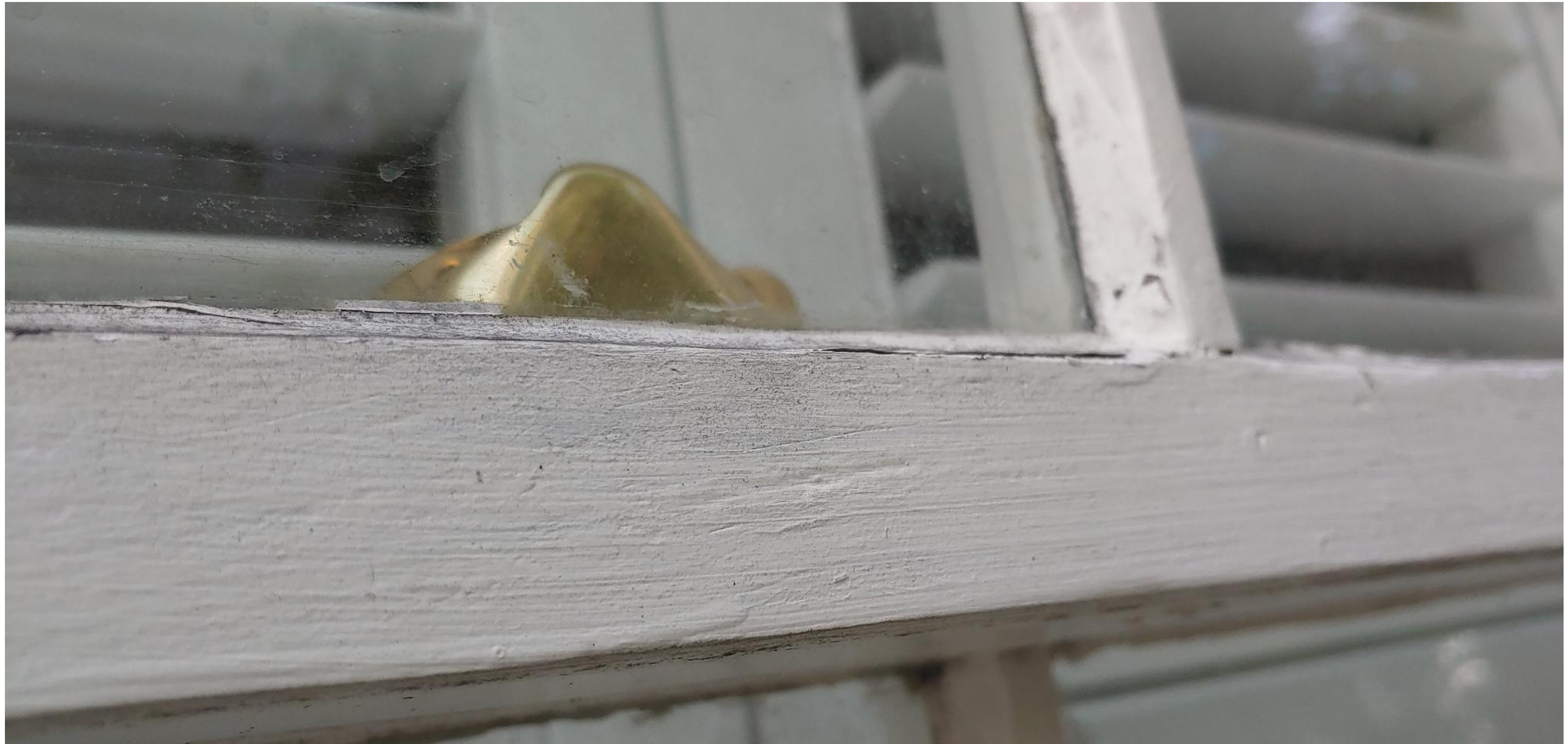
Up-close of Window Hardware on East Elevation. 1012 Southard Street. Photo by Brandon Celli.
