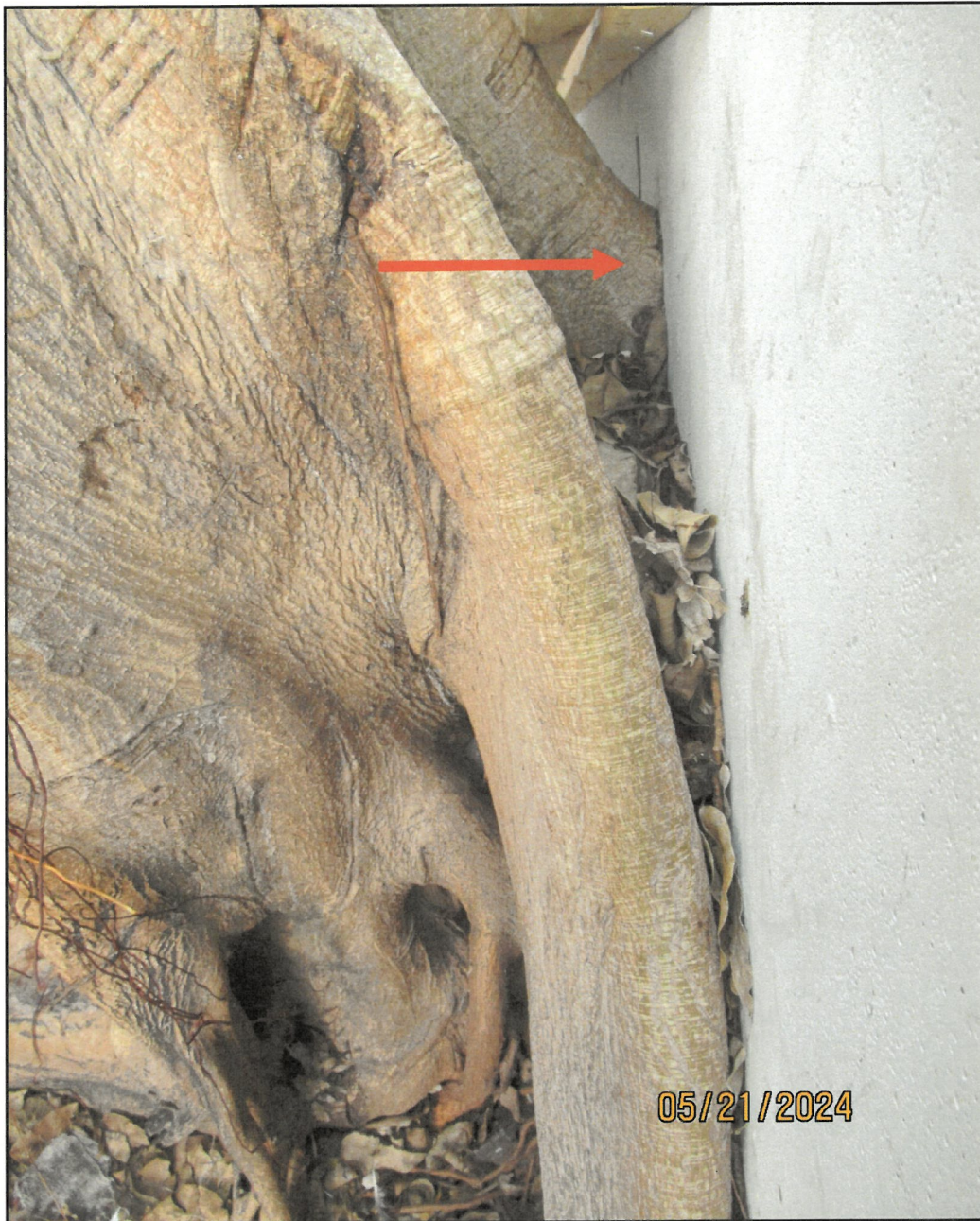
The roots of the strangler fig tree are growing into the base of the parking structure, pushing on the wall.
