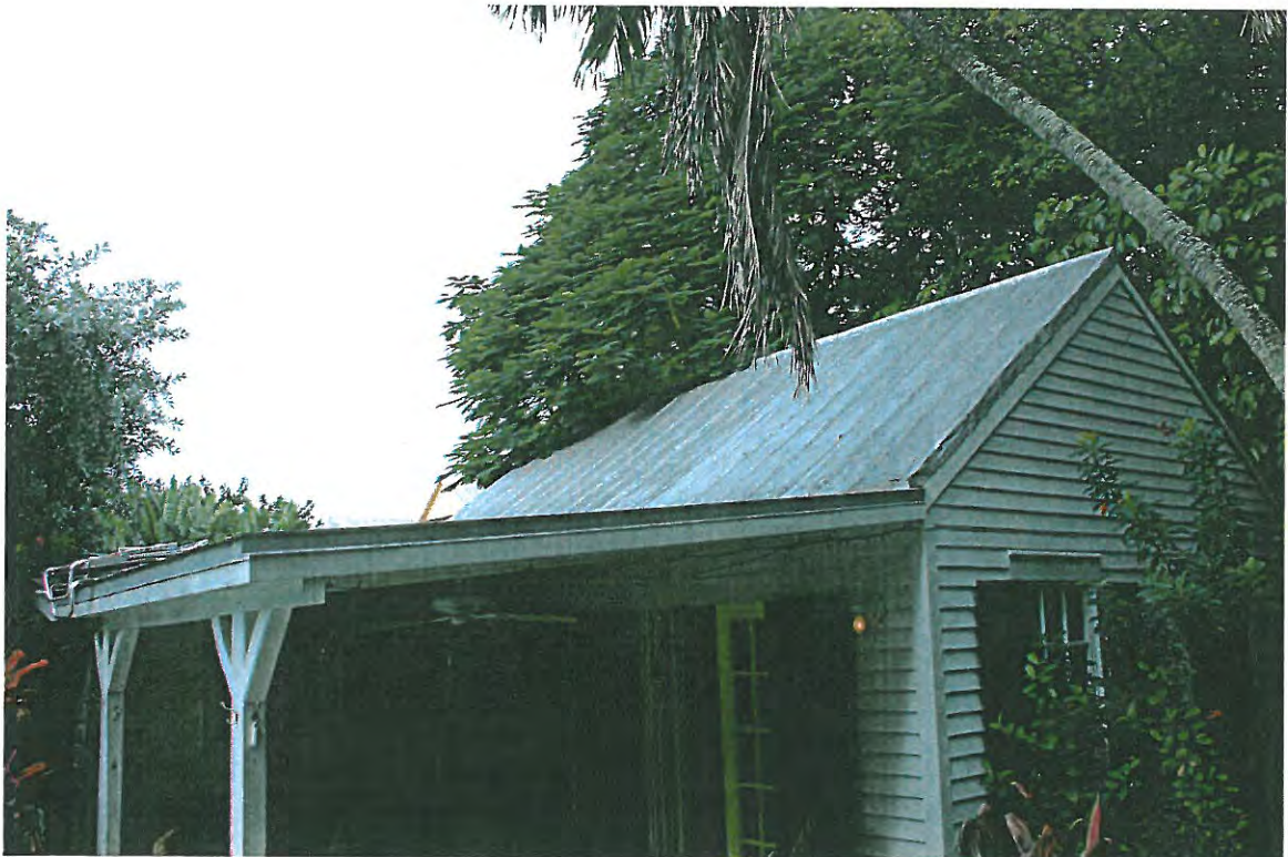
NEW SHED ROOF TO BE REMOVED
