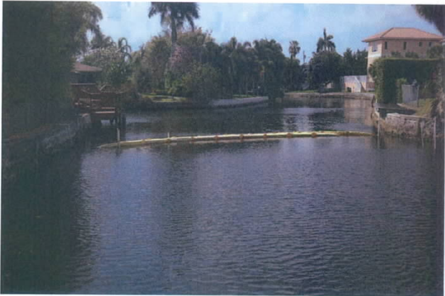
Coral Lakes typical section with turbidity curtains to prevent water quality impacts.
