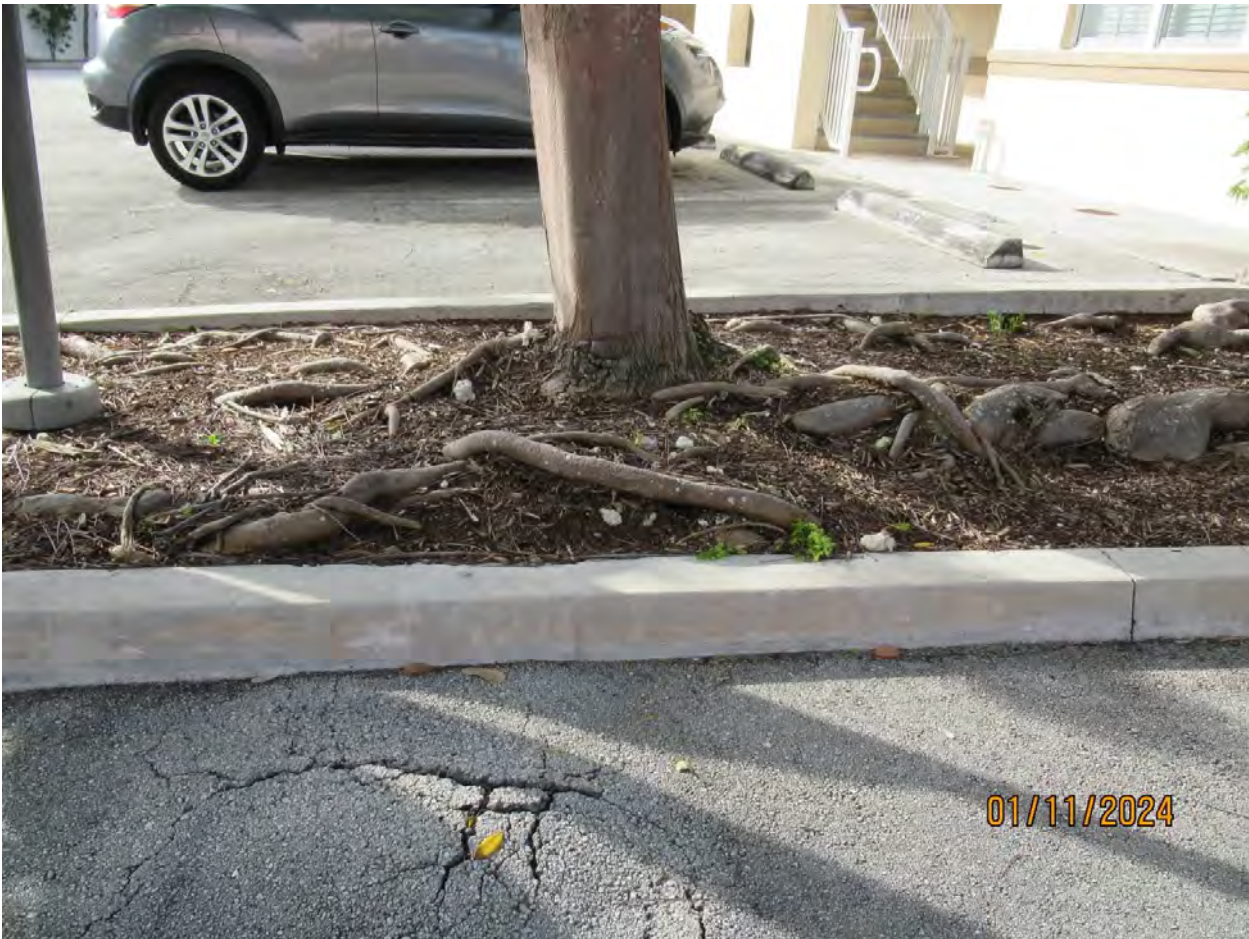
Two photos showing base of tree and root system related to parking lot area, view 3 & 4.
