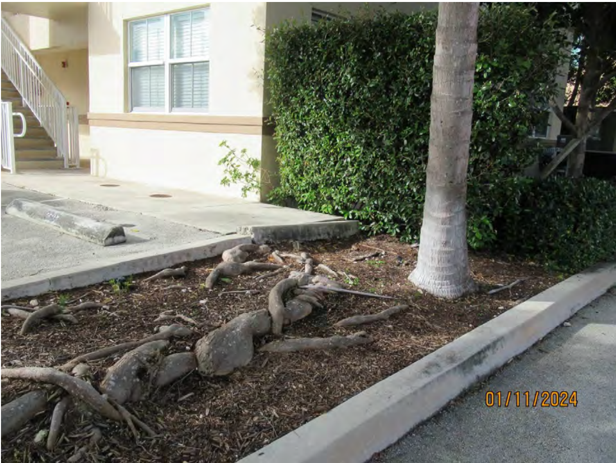
Photo showing tree root impacts with sidewalk curbing, view 2.
