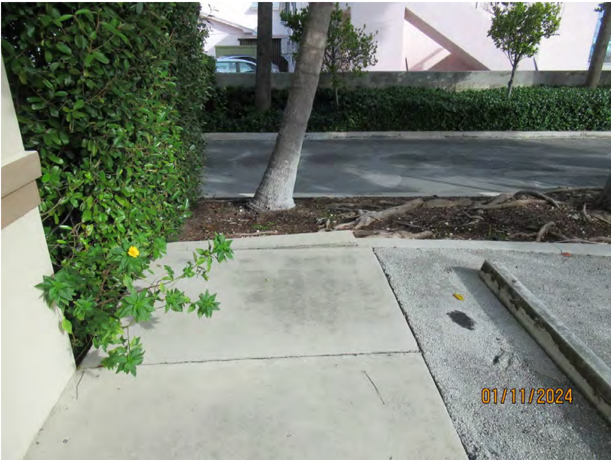
Photo showing tree root impacts with sidewalk curbing, view 1.
