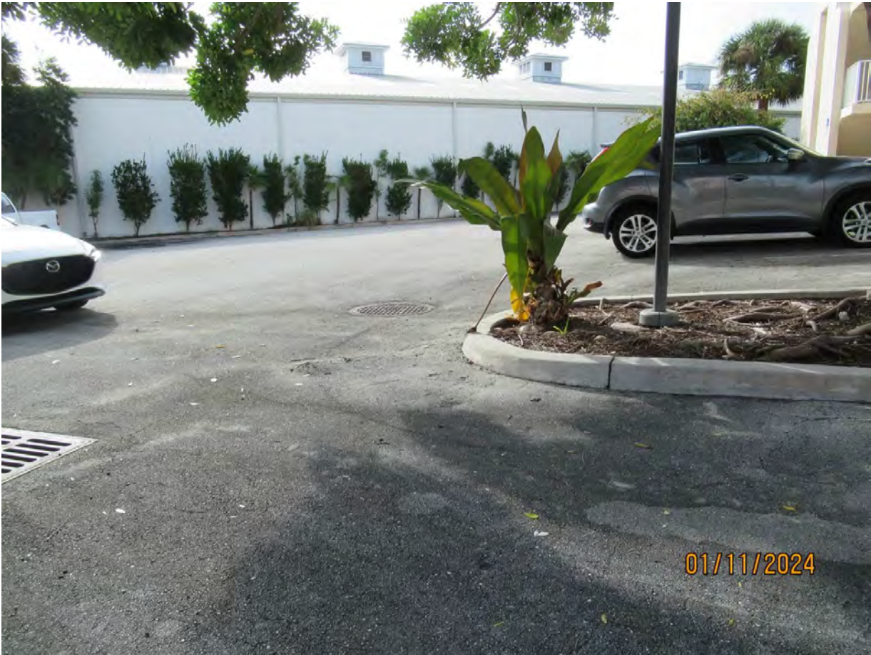
Photo showing root impacts to asphalt area near tree.
