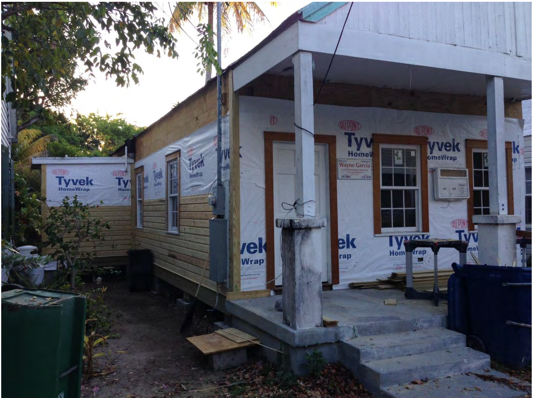
When staff went to assess the siding condition.
