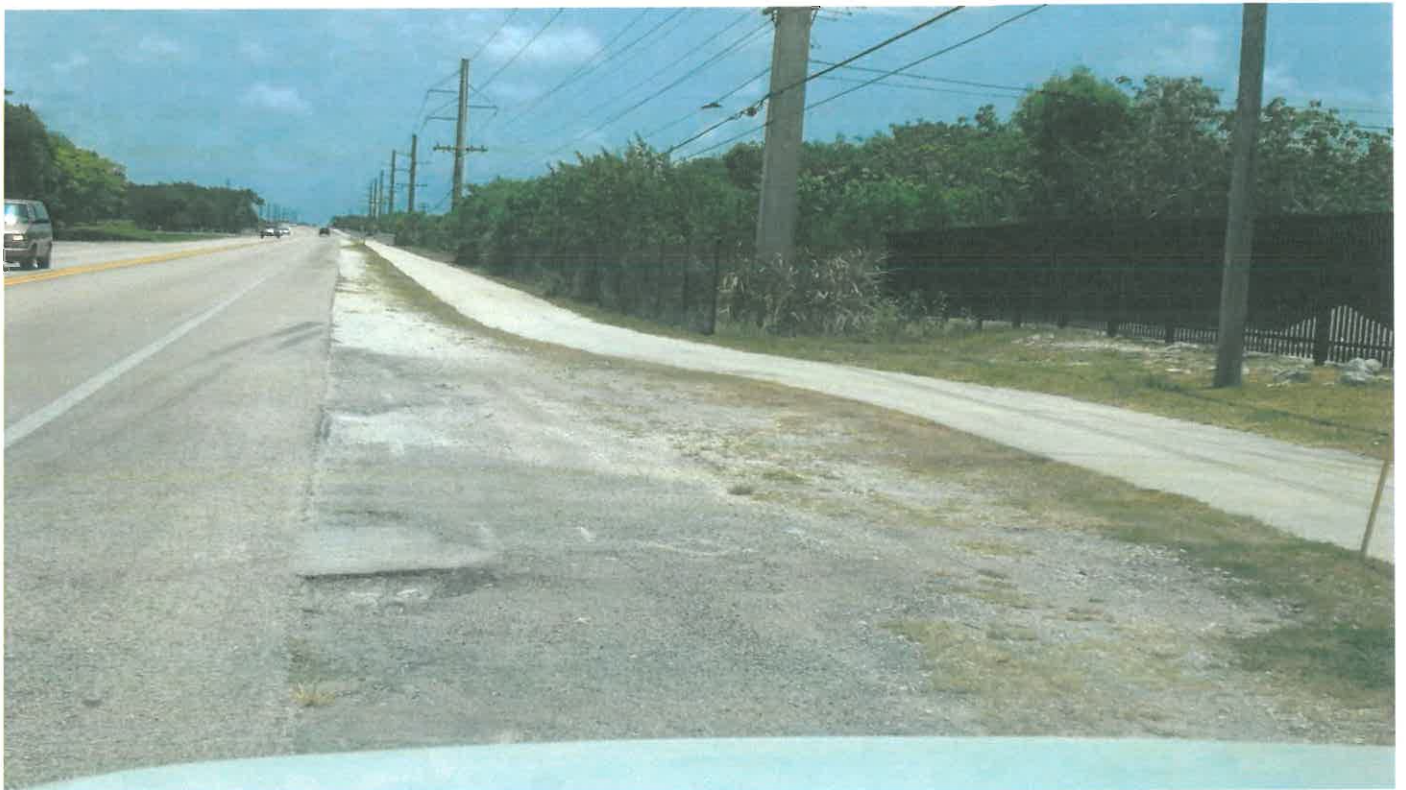
Just North of FKAA Pump Station – Ramrod
