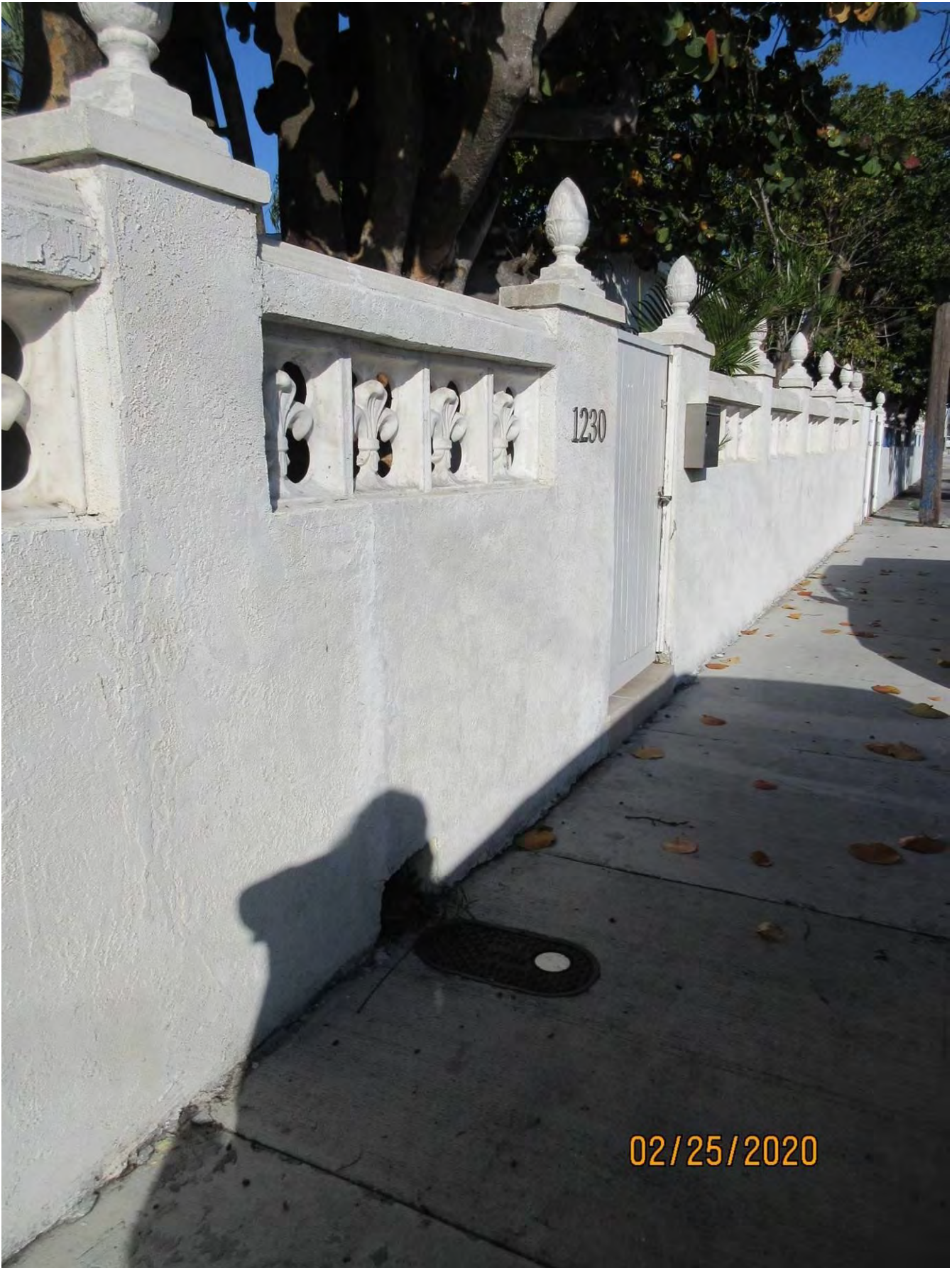
Photo showing location of water meter and tree. Also showing recently repaired cracks in wall, view 1.
