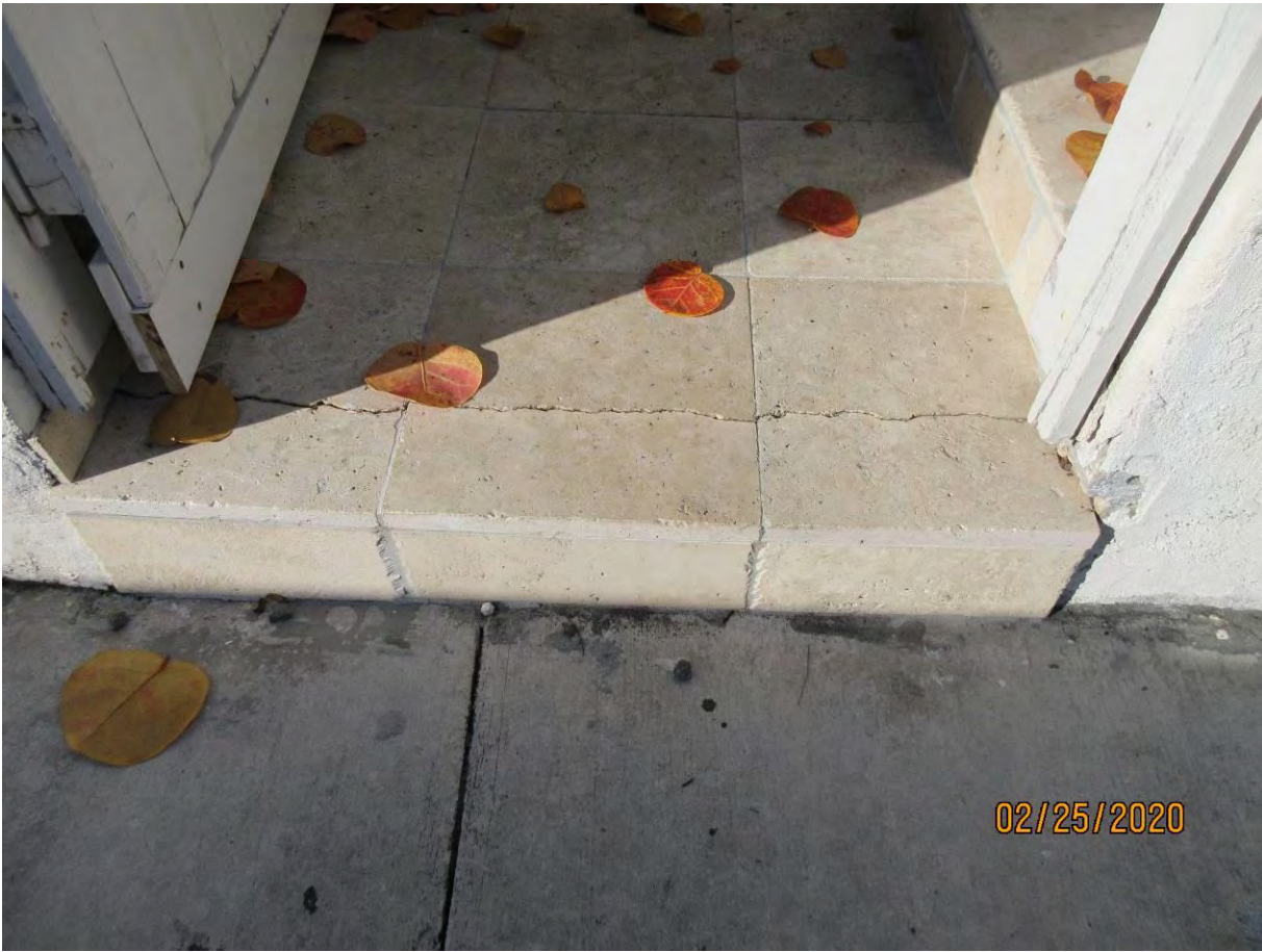
Photo showing damage to tile and entrance area.
