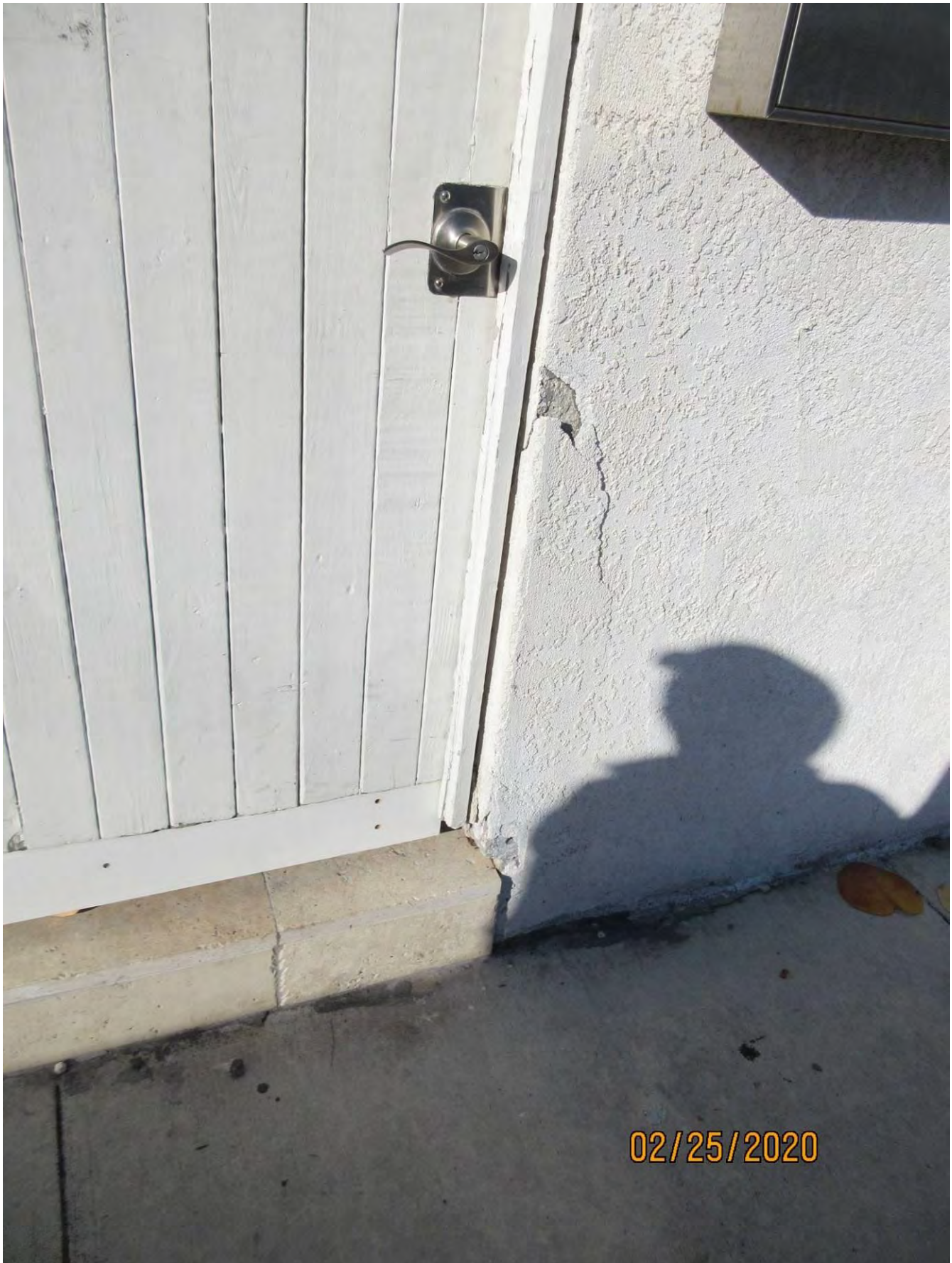
Photo showing cracks in wall and gate step, view 1.
