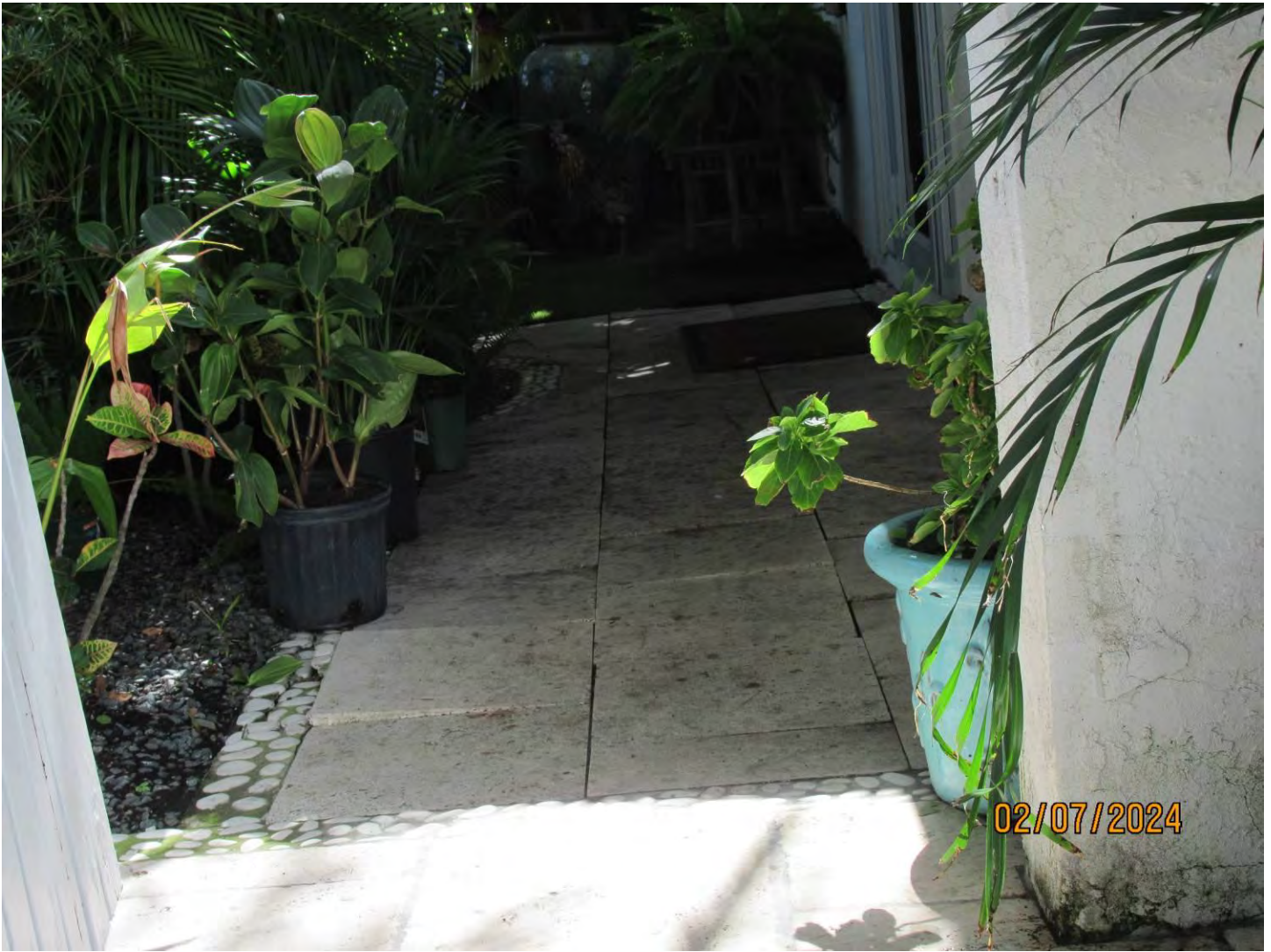
Photo showing uplifting of tiles in walkway.
