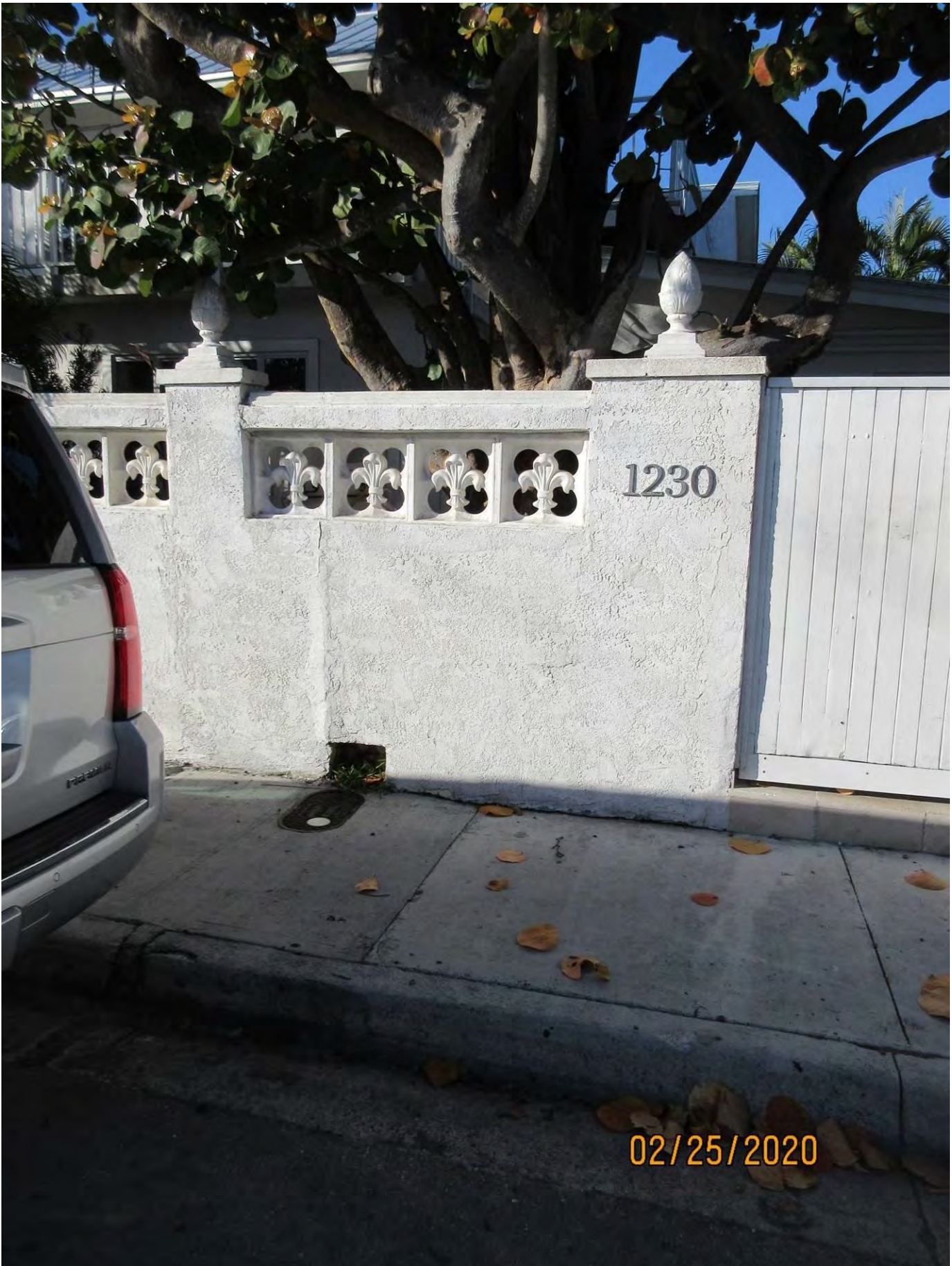
Photo showing location of water meter and tree. Also showing recently repaired cracks in wall, view 2.
