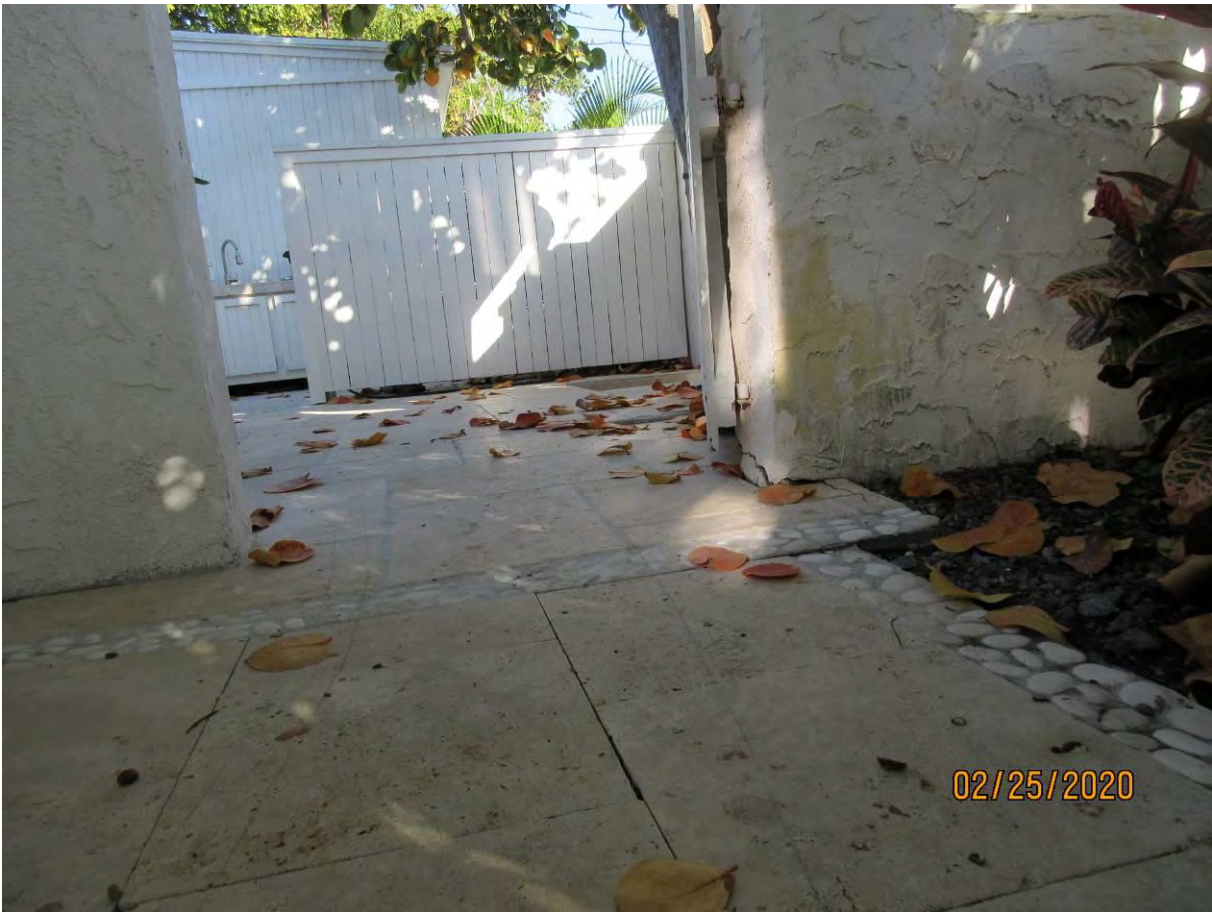
Photo showing interior walkway and wall area damage. Propane tank is located behind wall.
