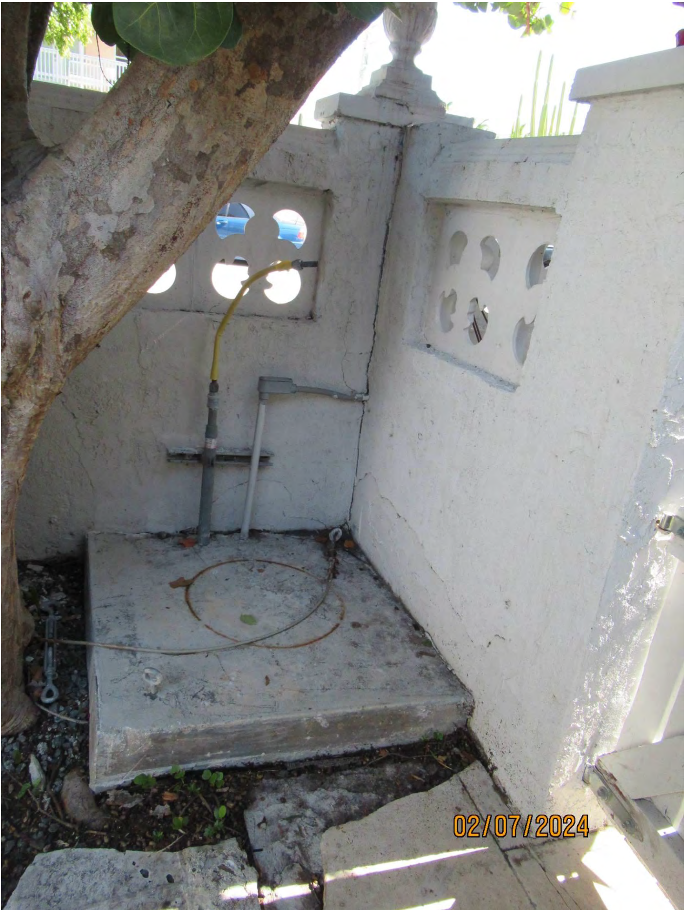
Photo showing cracking in fence/containment walls. Propane used to be installed in this area.
