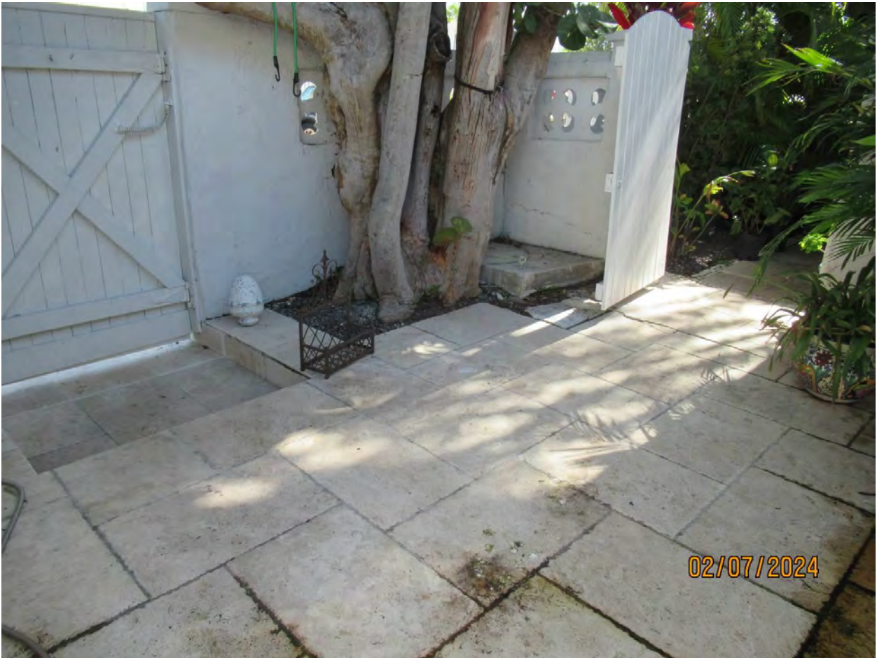
Two photos showing base of tree area and the surrounding impacts.
