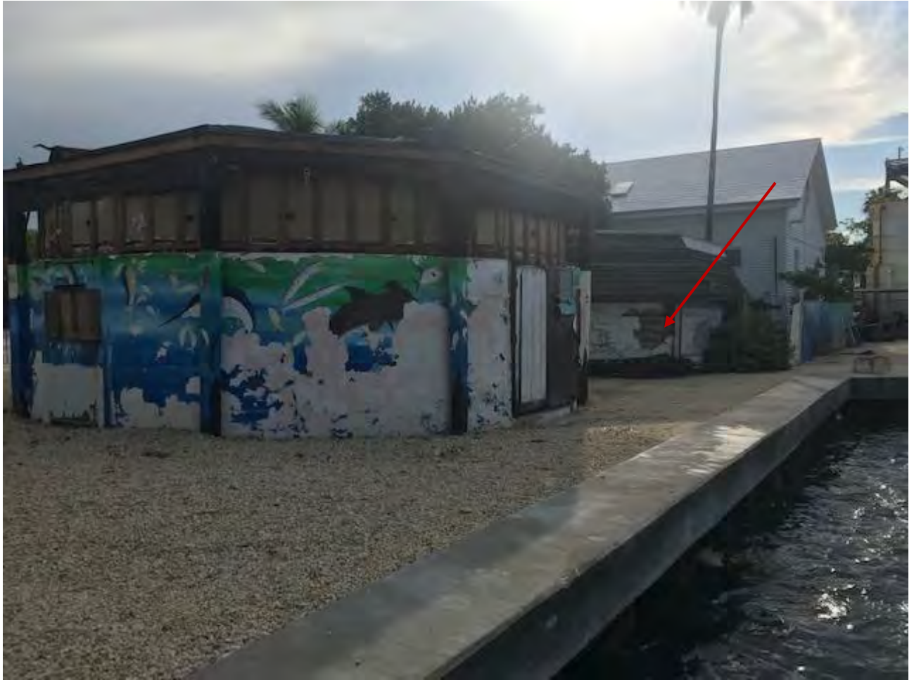
Rear of both Cable Huts. Notice spalling on the easternmost Cable Hut.
