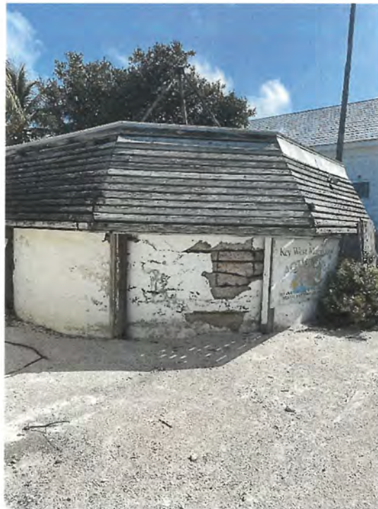
East Cable Hut showing spalling of concrete and horizontal slat roofing.
