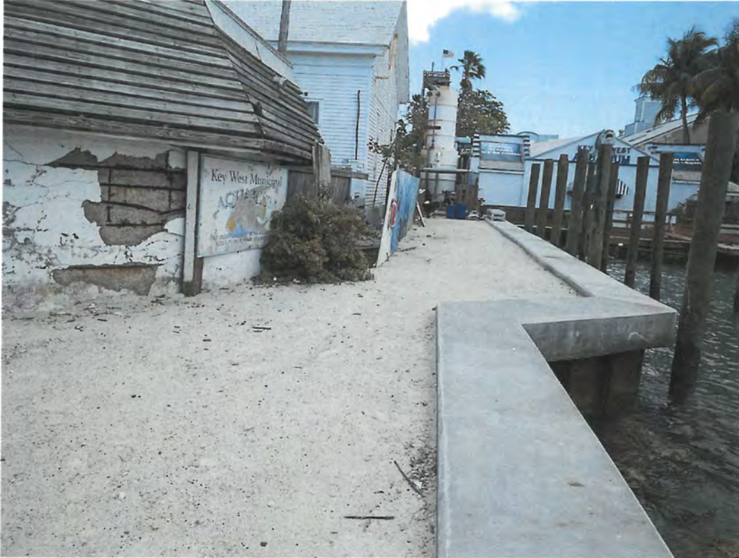
West elevation of East Cable Hut, the Aquarium is in the background.
