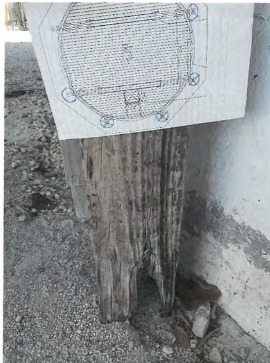
Deteriorated column at grade. All columns will be re-set in new foundations and repaired.
