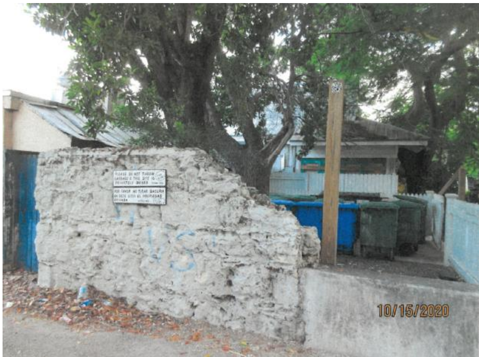
Site Visit – Photo depicts damaged wall that must be repaired or replaced with HARC approval for a new wall or fence.
