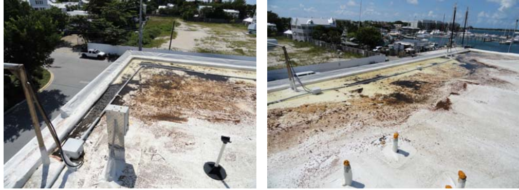
Photos 12 and 13 - Building Structure D Roof Ponding Water
