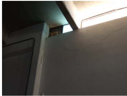
Photo 11- Building Structure B Damaged Column
