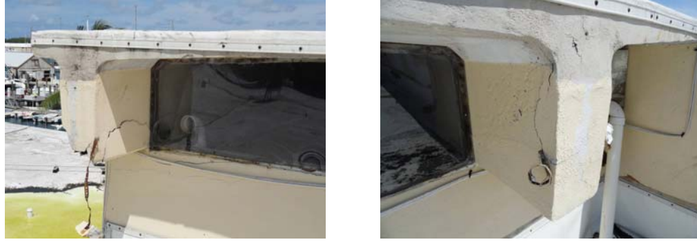
Photos 09 and 10 - Building Structure B Damaged T-section
