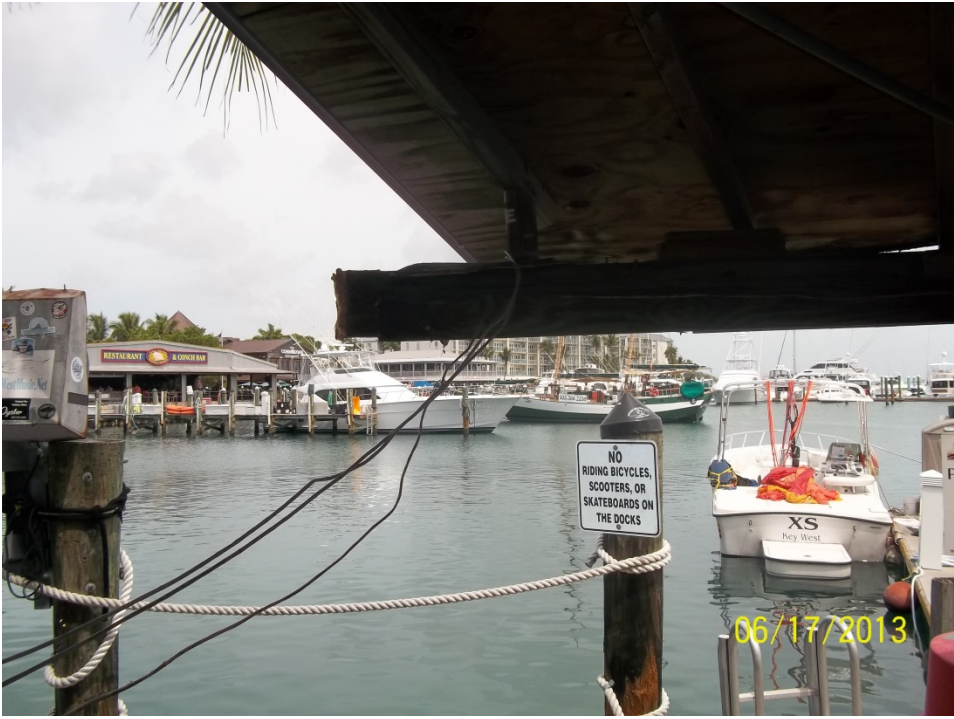
Schooner Wharf. Wall removed without the benefit of a building permit or HARC Certificate of appropriateness
