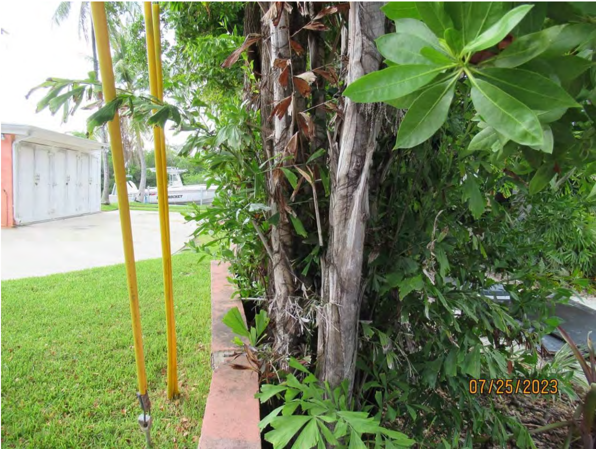
Photo of the trunk area of tree #1 & #2 and the property line wall.
