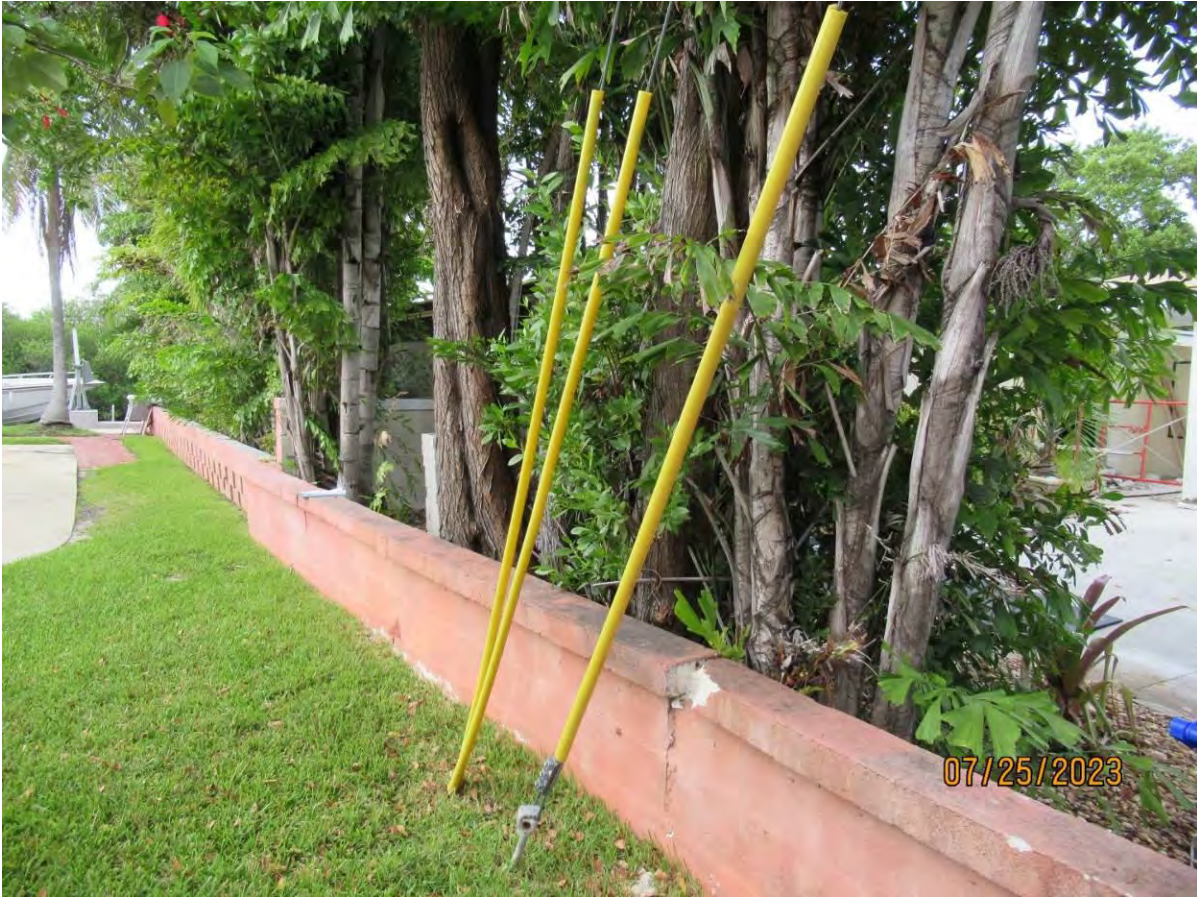
Photo showing base and trunk areas of trees 1 & 2 and the property line wall.
