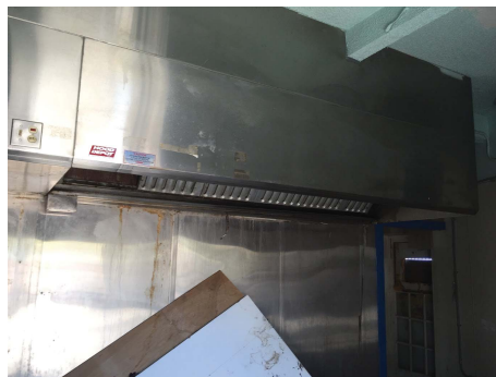
EXISTING CABLE HUT INTERIOR REMOVE ALL INTERIOR KITCHEN EQUIPMENT & NON HISTORIC MATERIALS
