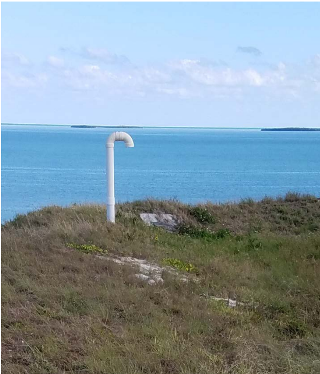
Typical gas vent (GV).
