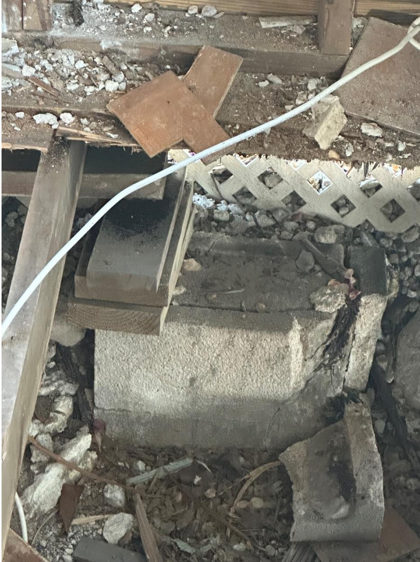
Photograph 6: Another photograph showing the foundation and damaged framing.
