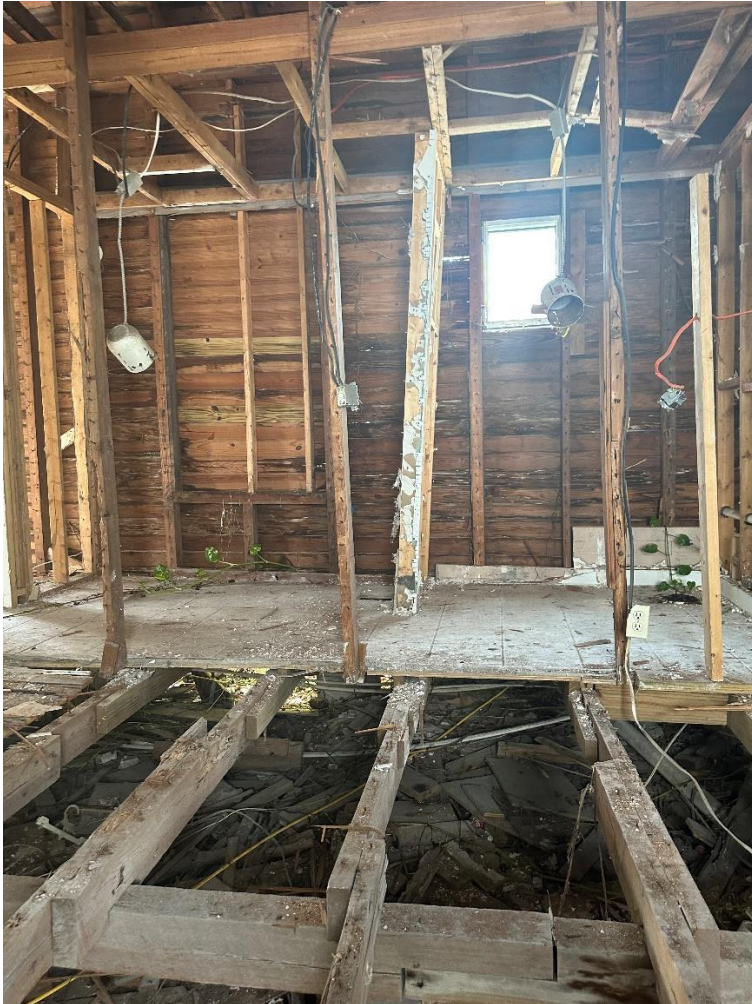
Photograph 1: View of the interior of the structure. The beam is not supported and the wall studs are damaged as well as the window.
