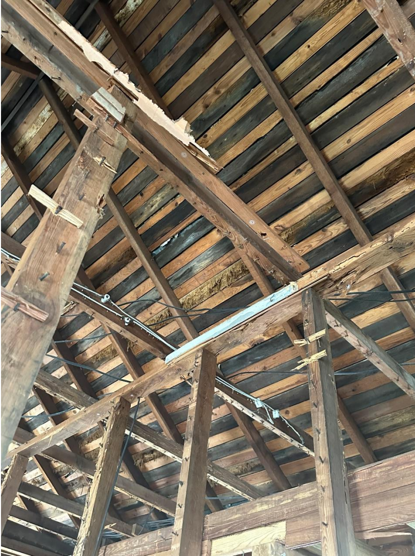
Photograph 5: Photograph of the undersized rafters and damaged wall framing.
