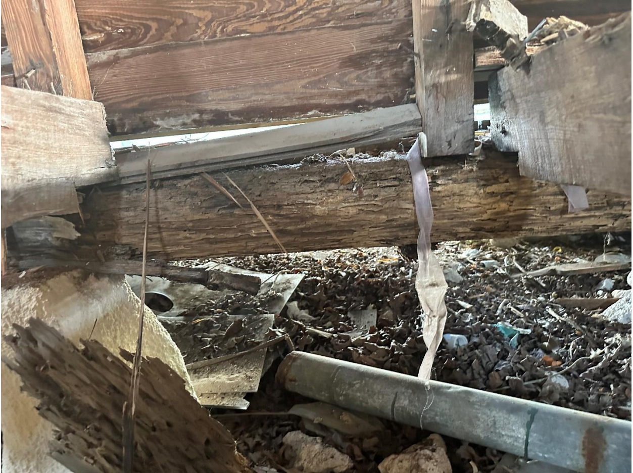
Photograph 7: Photograph of the damaged rim beam, eroded column and damaged studs and siding.
