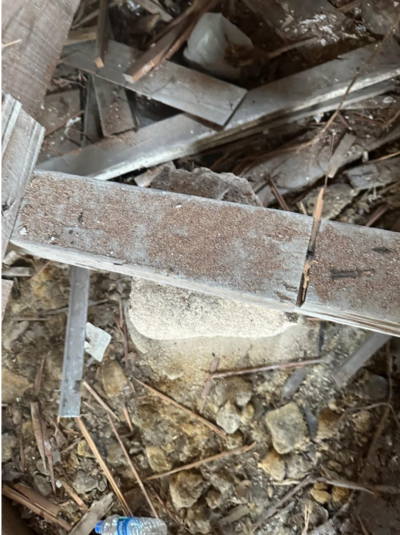
Photograph 2: View of eroded column with no tie downs and termite damaged beam.
