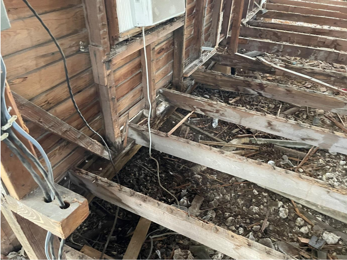
Photograph 3: View of the termite damaged rim beam, joists and studs.
