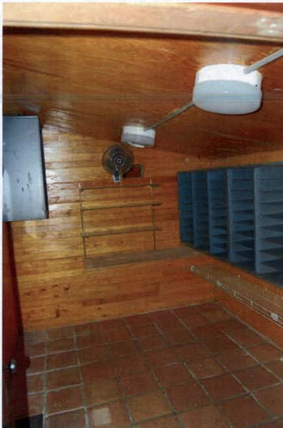
View of interior of non historic addition. The floor is 5" below the historic structure. This is a shed roof which terminates at roughly 6'-0" above the finished floor level.
