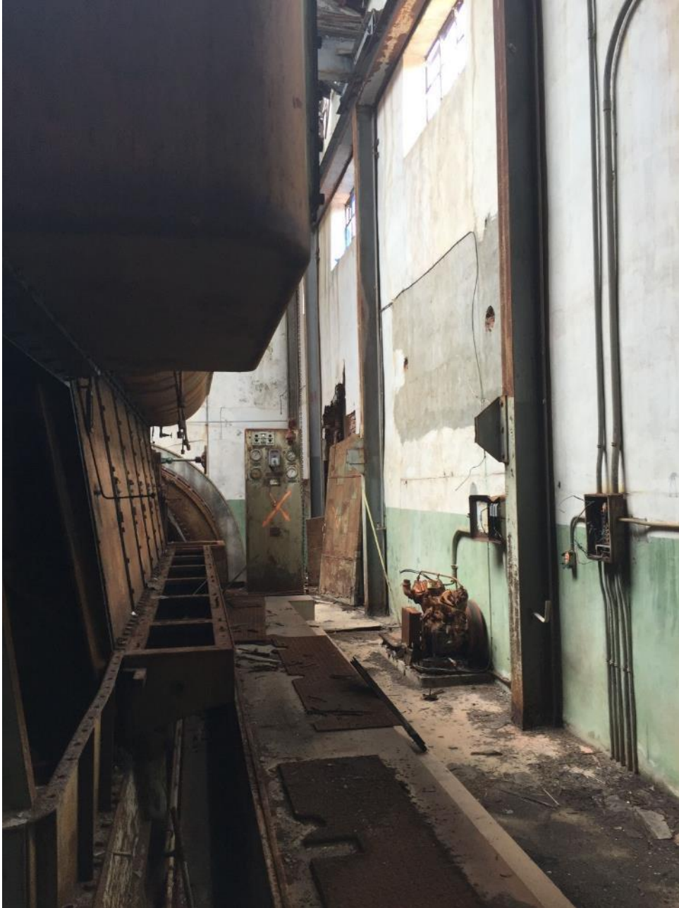
PHOTO 3: Inactive generator inside buildings at the Site
