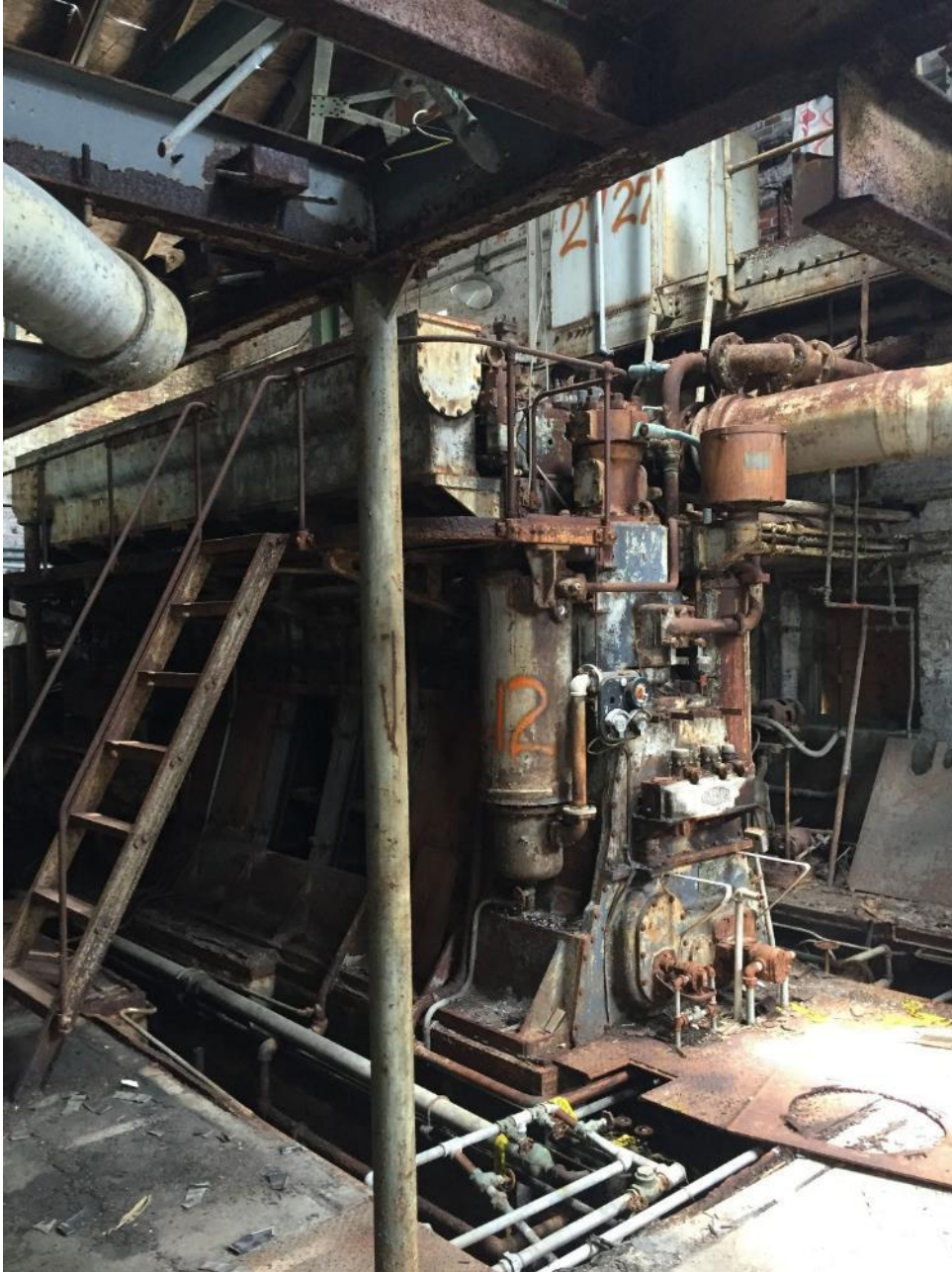
PHOTO 2: Inactive generator inside buildings at the Site
