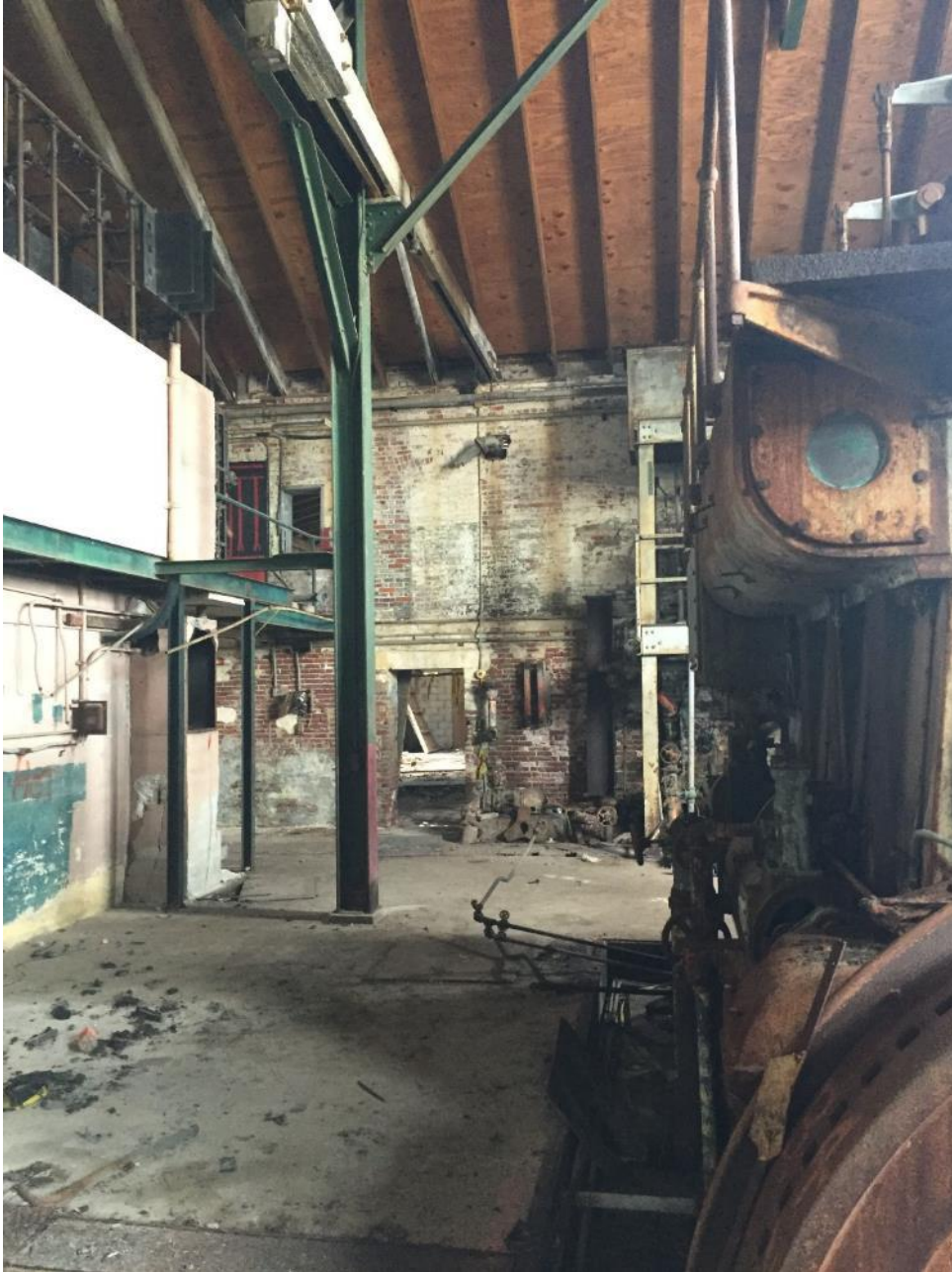
PHOTO 8: Interior of buildings at the Site showing an inactive generator
