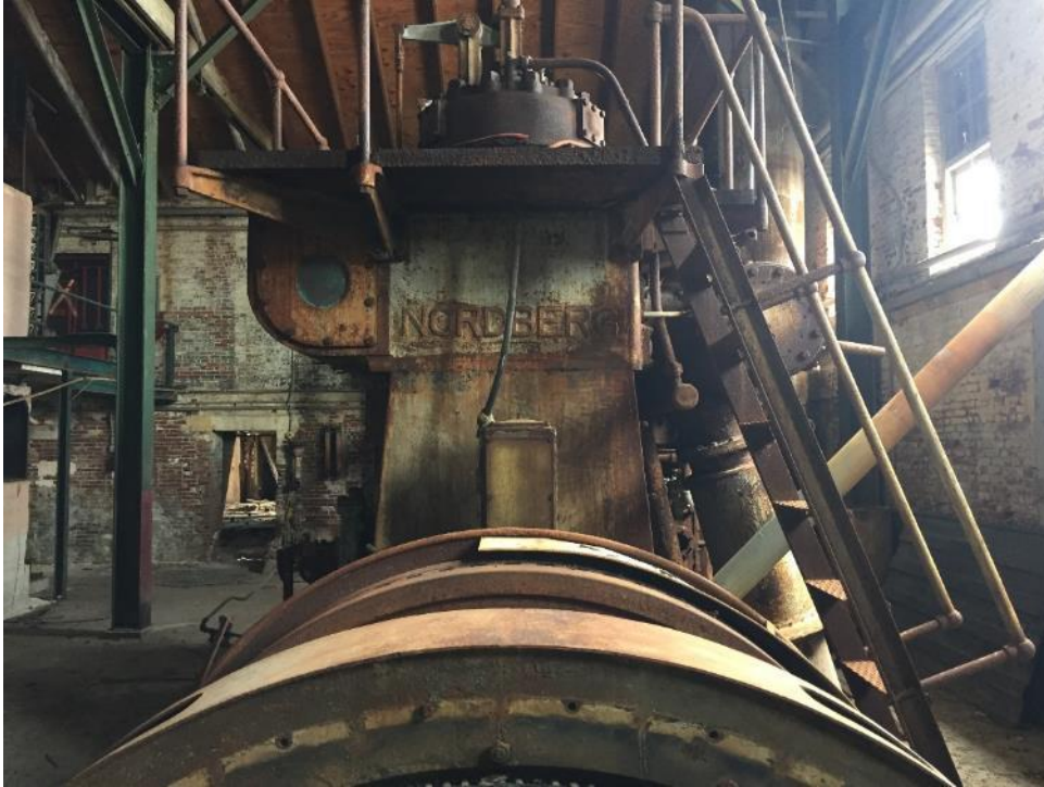
PHOTO 9: Interior of buildings at the Site showing an inactive generator
