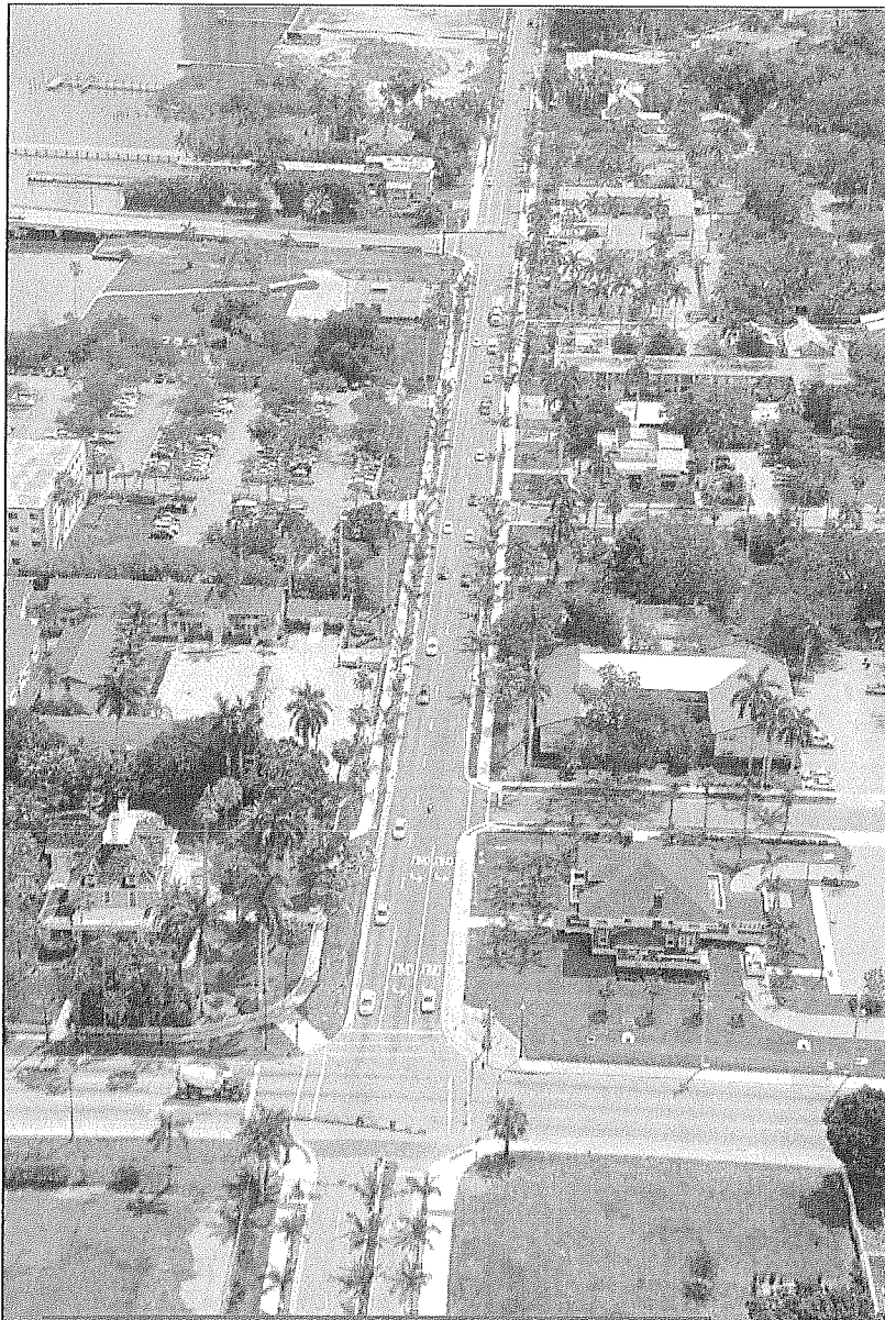
Above: State Road 80 (1st Street) in Fort Myers Looking West Right: Drainage Installation.
