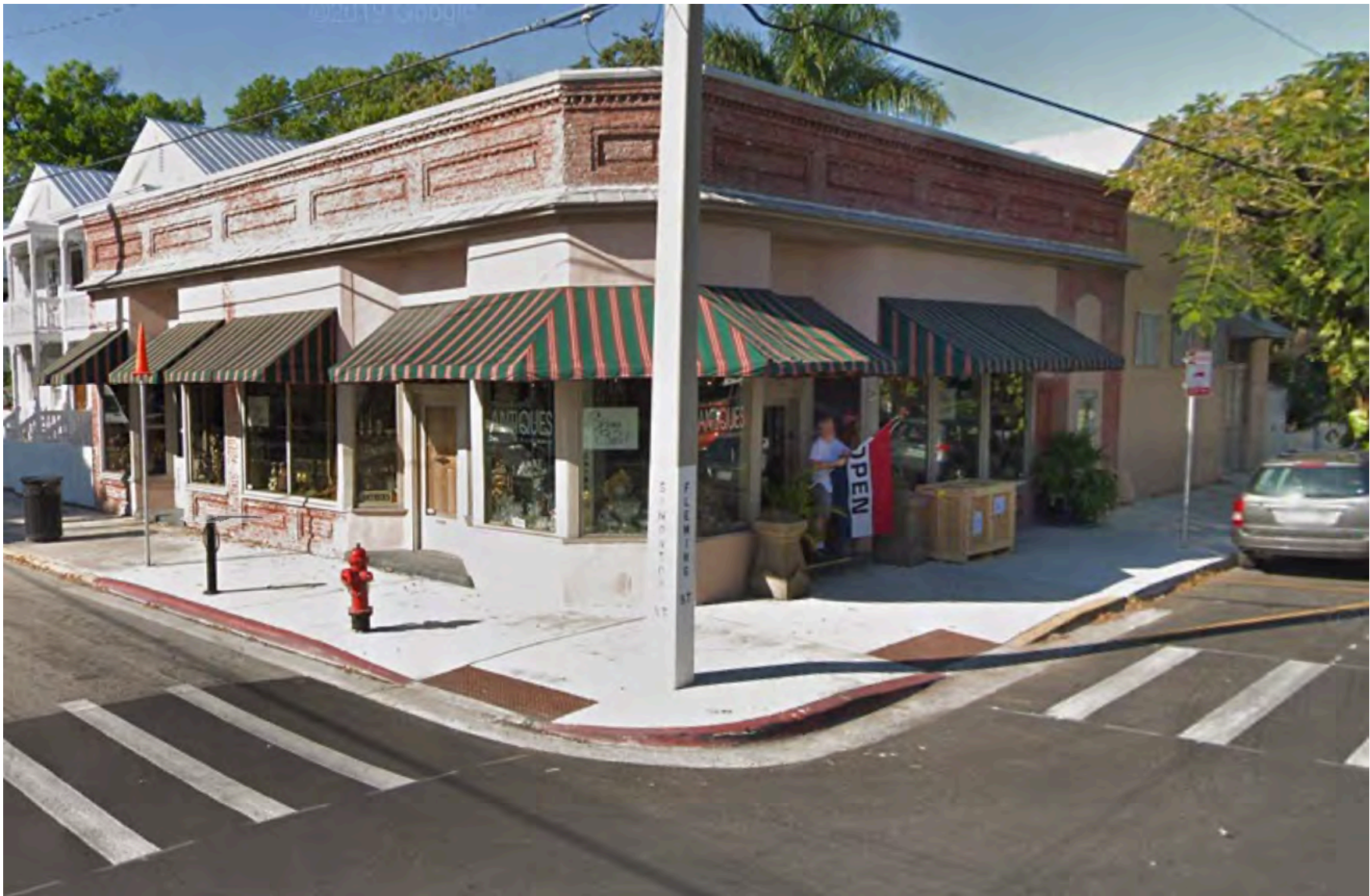
Example of historic brick building in historic Key West with similar stucco repair
