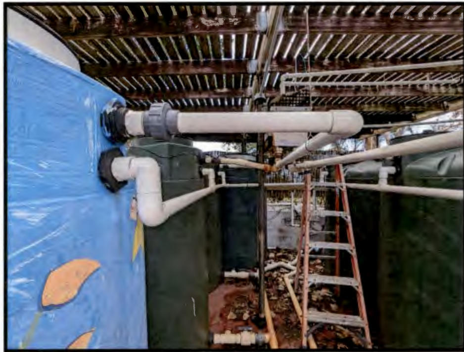
EXISTING SEVEN 500 GALLONS INTERCONNECTED IRRIGATION TANKS
