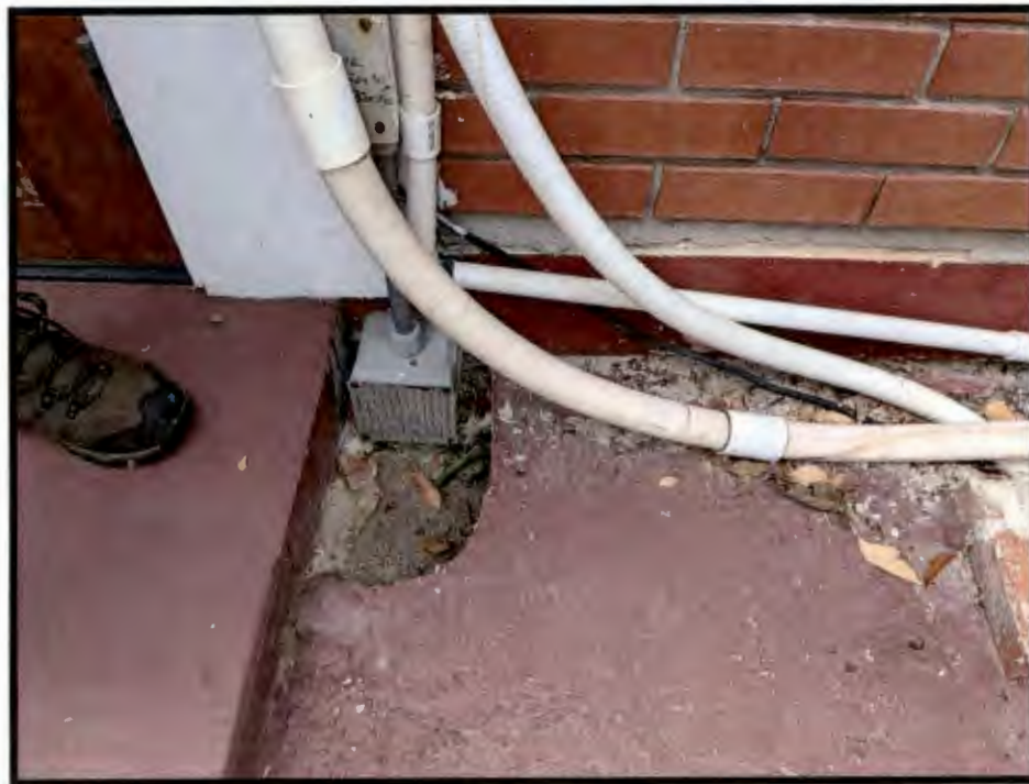
EXISTING PUMP#2 WATER LEVEL SENSOR
