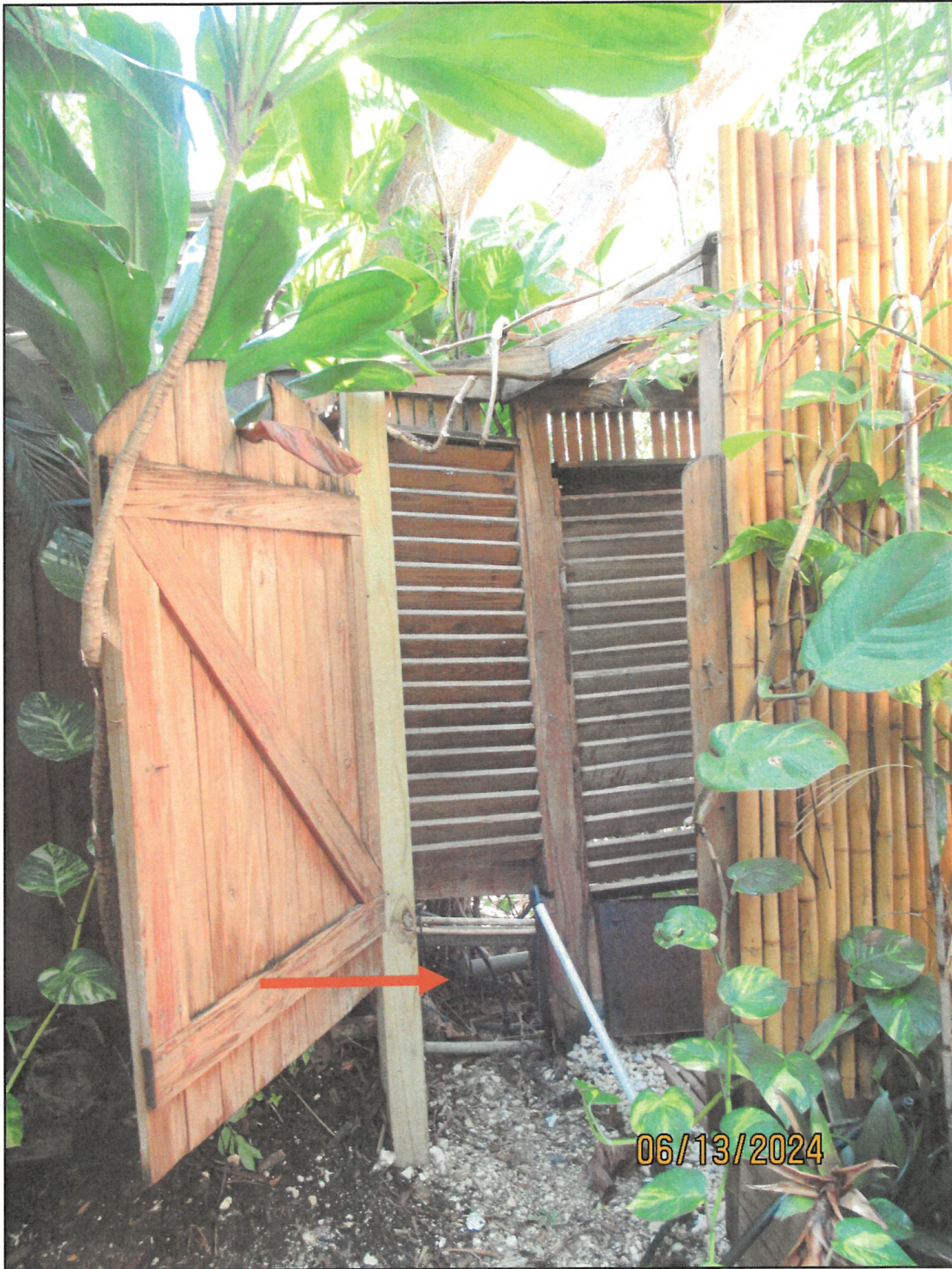
The roots of the gumbo limbo have damaged the wooden fence between properties and the outside shower walls.
