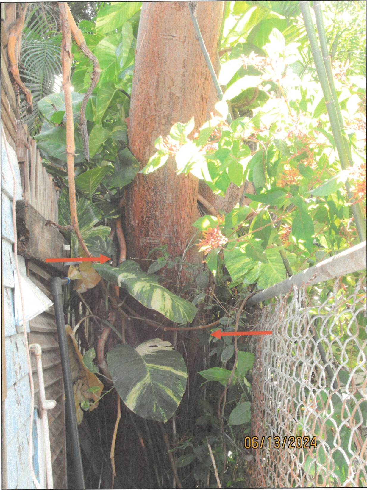
This tree was a volunteer between two fences and should have been removed at its sapling stage.
