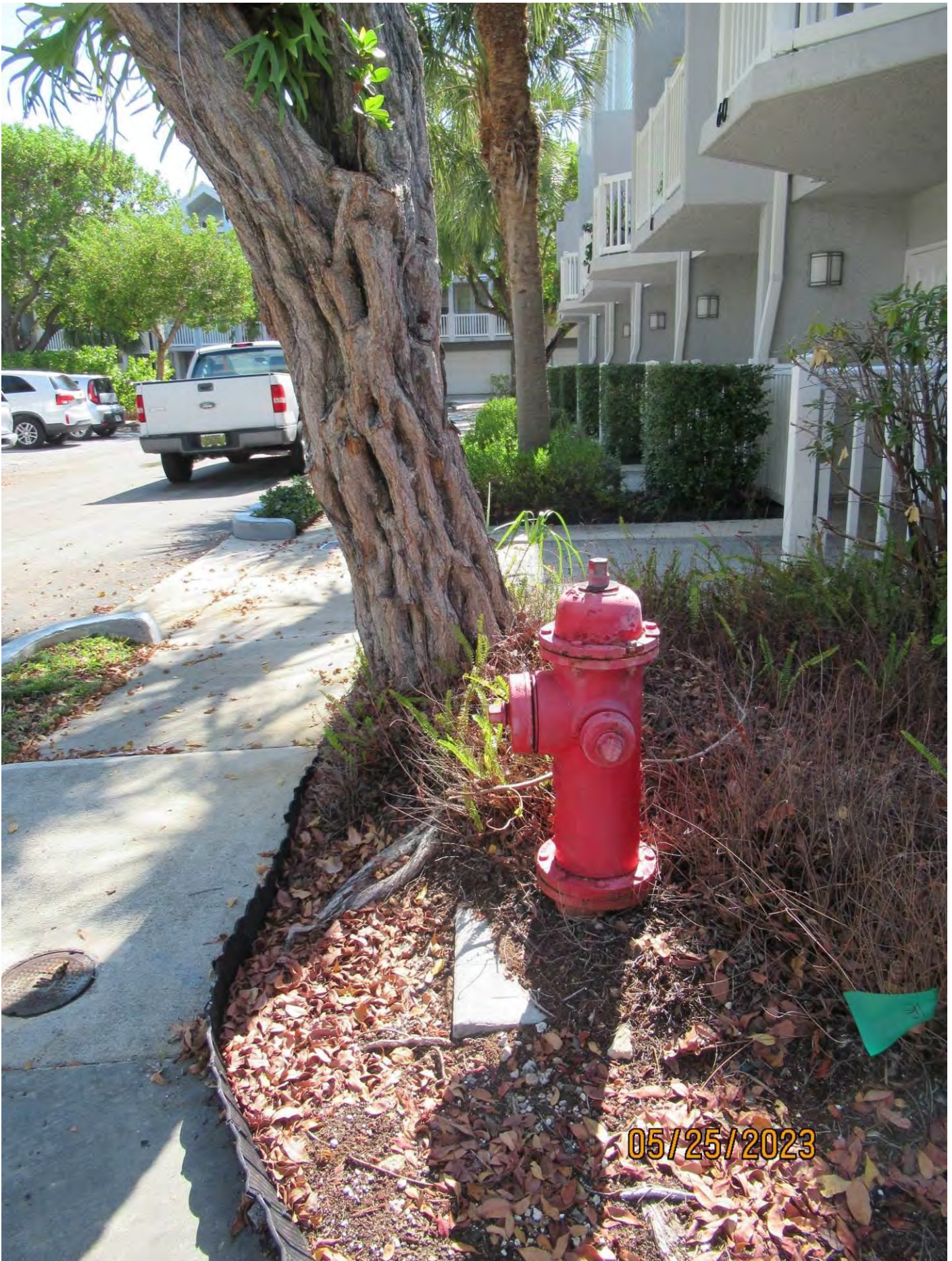
Photo showing tree root impacts to surrounding area, view 3.
